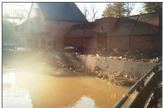
Photo: During the flood huge amounts of debris accumulated against the screens at the Foss Barrier, putting the pumps at risk of overheating
