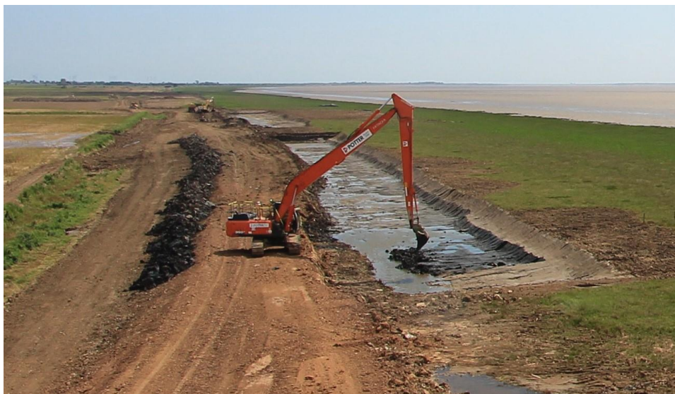
An excavator digging out the first part of the breach on the saltmarsh
