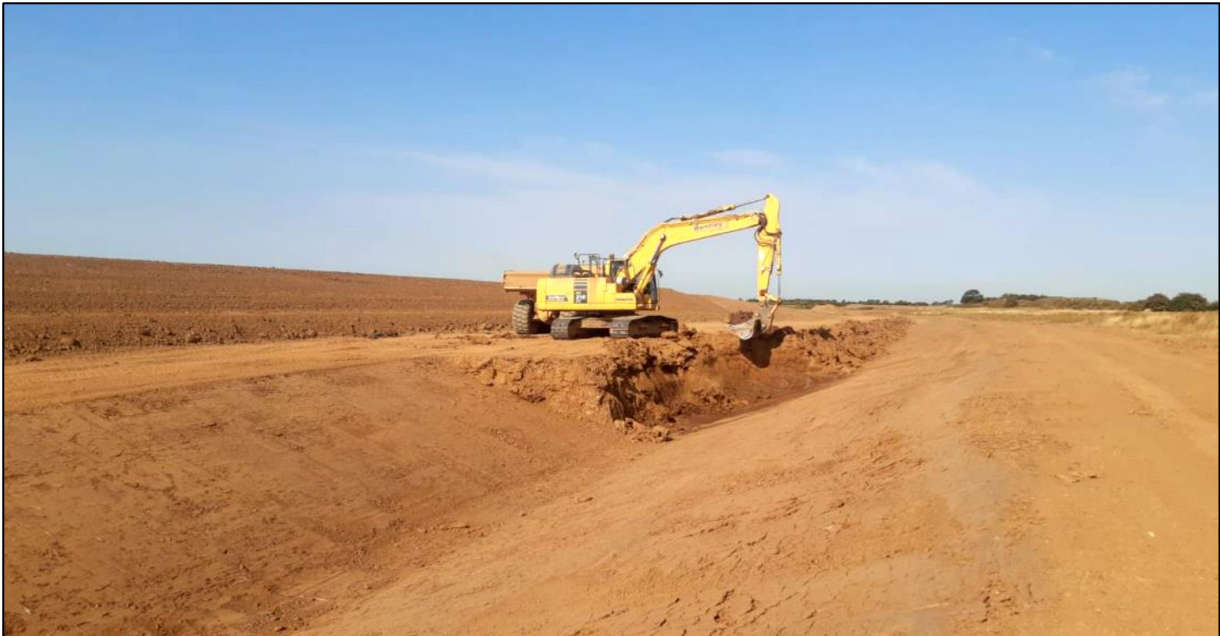
Photo: excavation of the new drain and flood embankment on the eastern side
