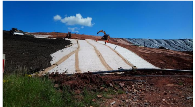
Above: Permanent capping placed with temporary plastic capping to the right of photo.
