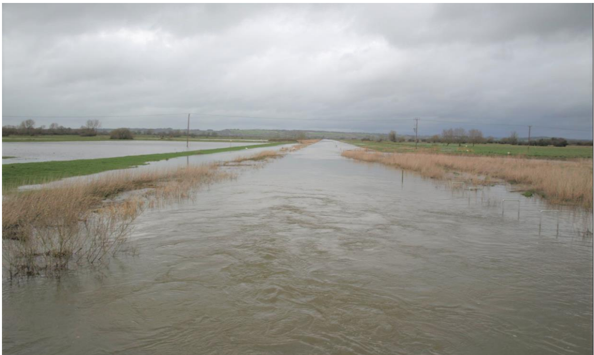
Figure 9.8 Photo Viewpoint 04 - View of the Sowy downstream of Beer Wall, illustrating the inconspicuous nature of the existing flood embankments
