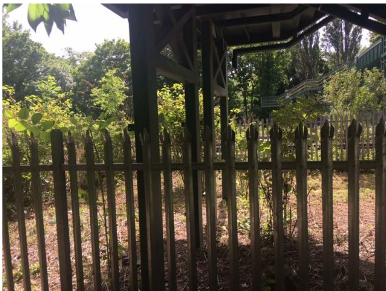
Photo 5: Japanese knotweed within rail foot bridge.
