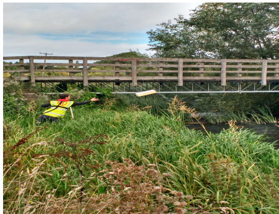
Plate 2: Installation of water vole floats, near Devils Backbone bridge, Oxford. Access down to bank restricted by vegetation and soft ground.
