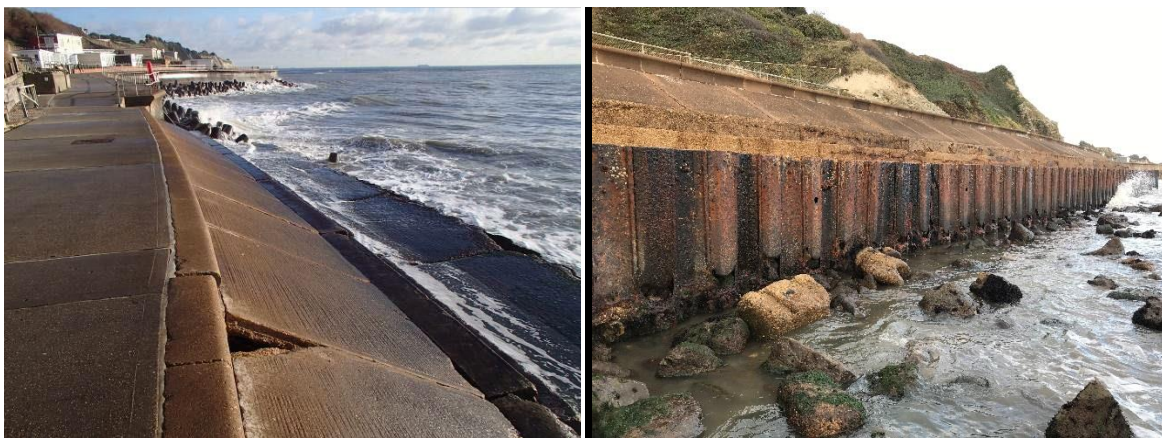
Images showing deteriorating coastal defences to the east of Ventnor, constructed in the 1970s.
