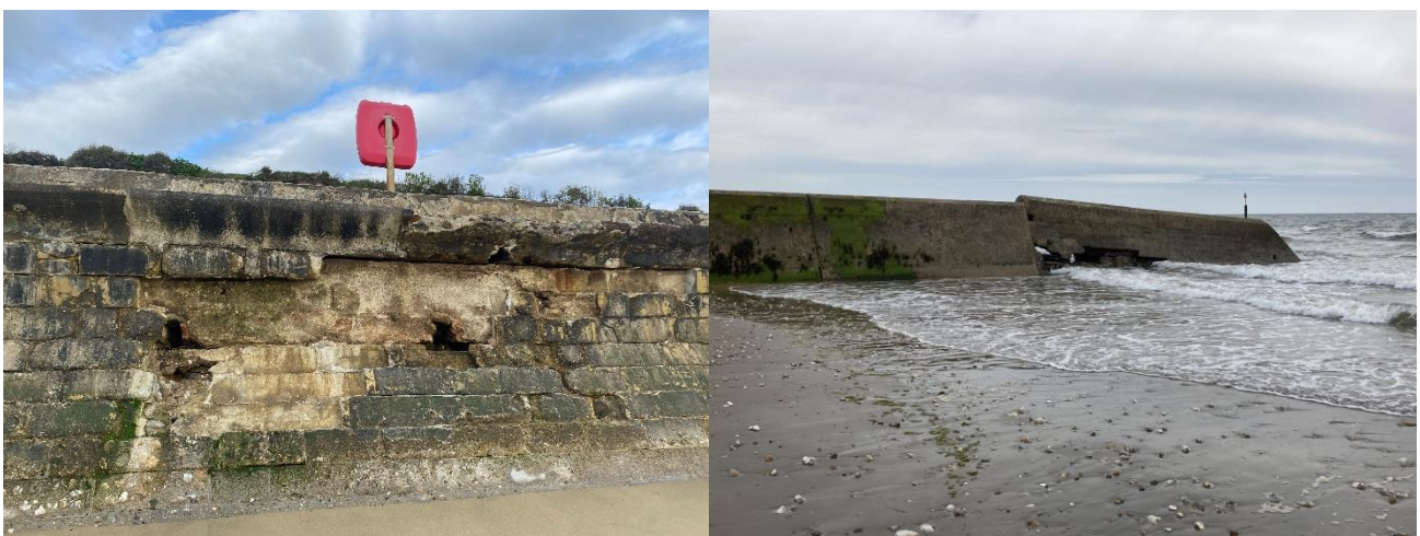
Figure 3 - Poor condition of the existing sea wall (left) and failed Hope Groyne (right)
