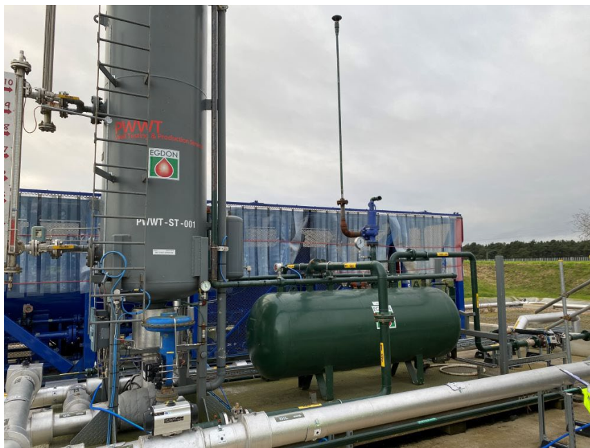
Figure 15: Typical process separation equipment (courtesy of Egdon Resources UK Ltd)
