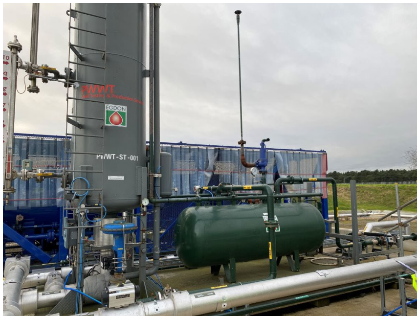
Figure 17: Typical process separation equipment (courtesy of Egdon Resources UK Ltd)
