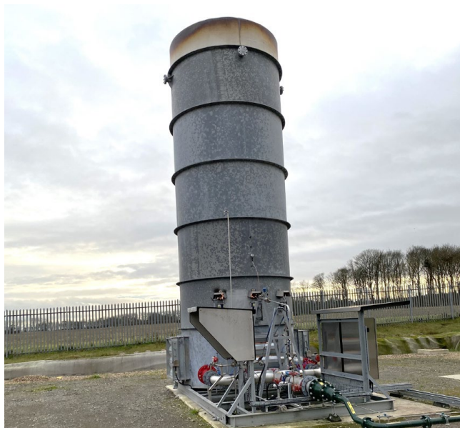
Figure 13: An example of a ground flare that may be used during ongoing testing and appraisal.
