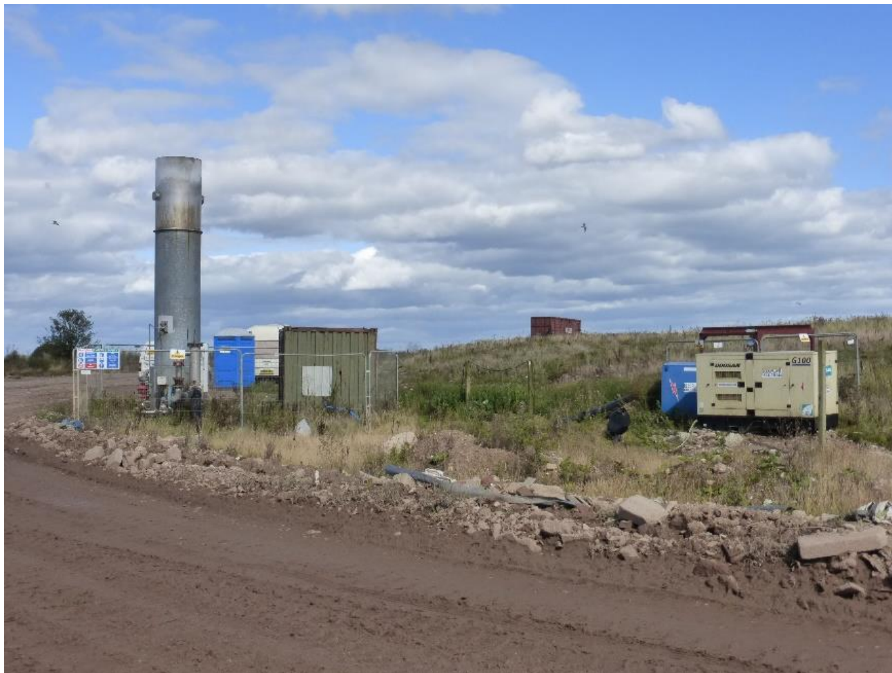
Figure NTS4: Current Landfill Gas Flare in Northwest Corner of Existing Site
