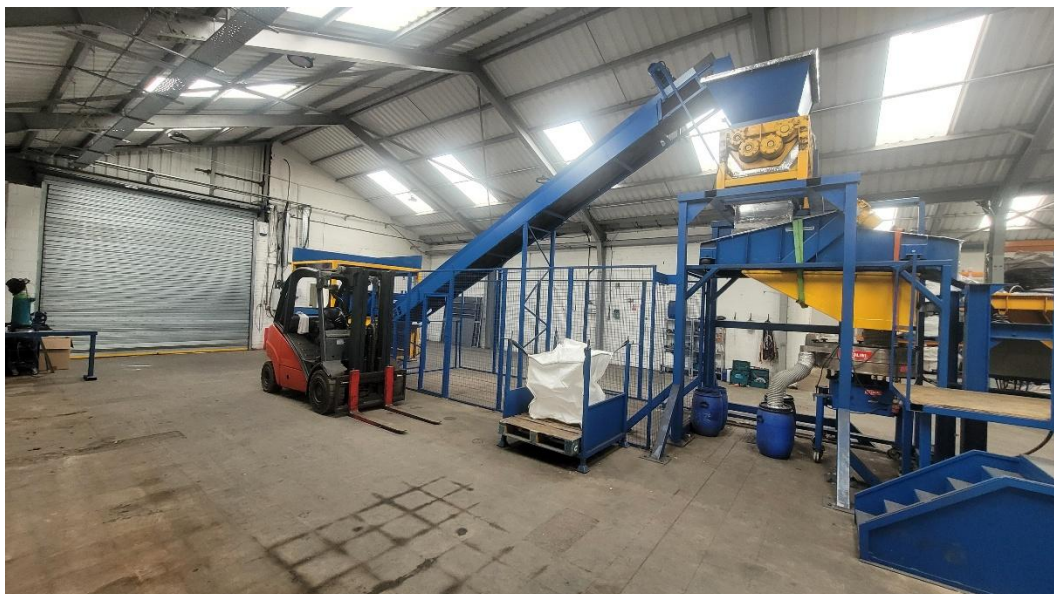
Plate 1 – Battery Processing Line– Looking Towards Northern End of the Processing Building
