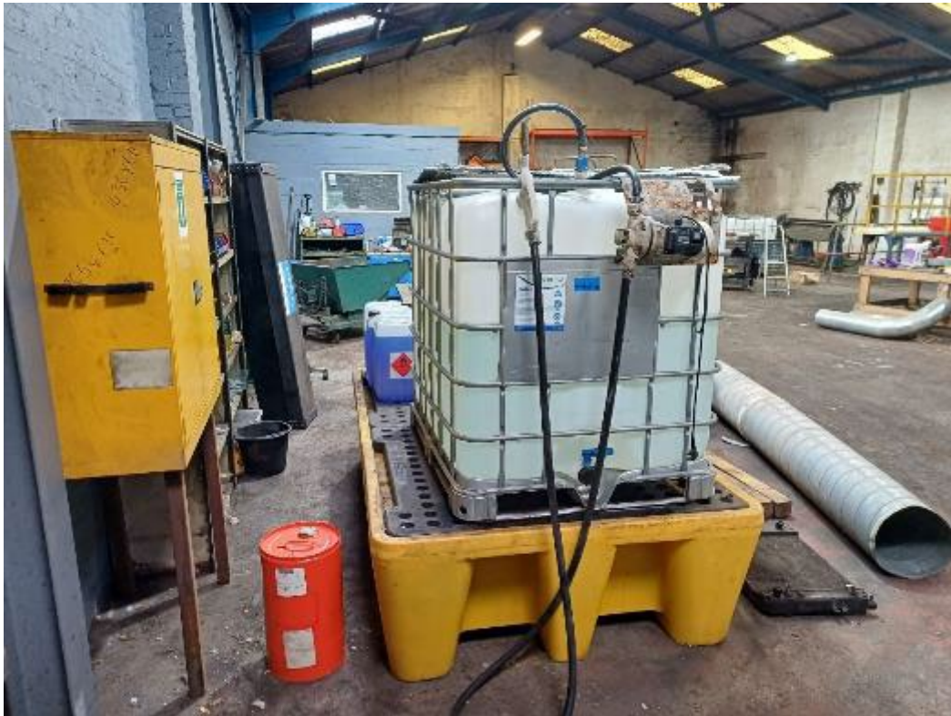
Photograph 11: Ad Blue stored on bunded pallets in the Maintenance Room within the internal Additional Area.
