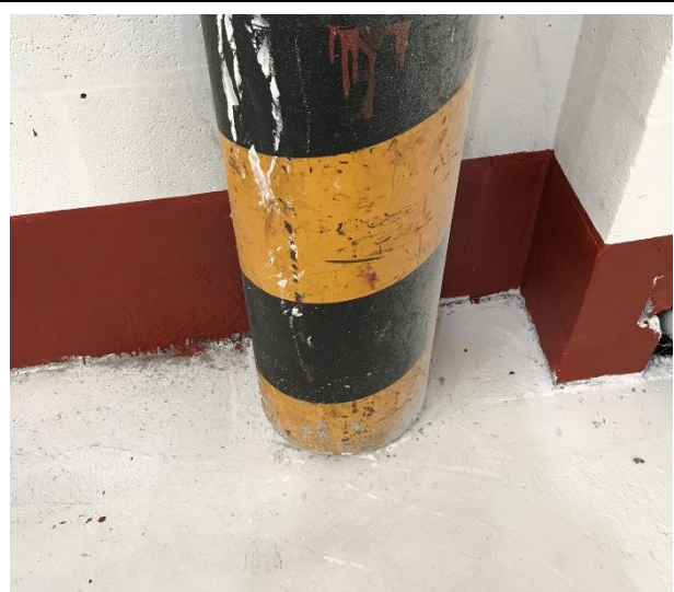
Sealed and protected internal downspout
