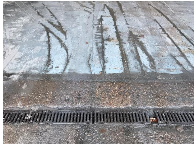
Aco grating into fabrication area.
