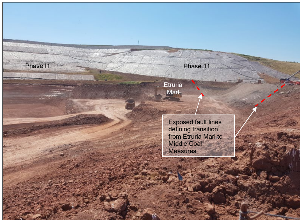
Figure HRA2: Exposed fault line on the western edge of Phase G2
