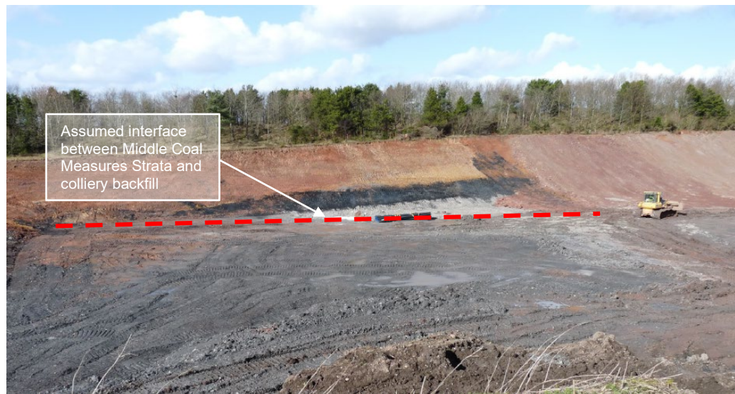
Figure HRA1: Extent of the Middle Coal Measures Strata across the base of the PFA Monocell
