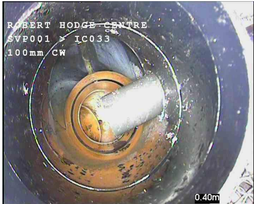
1, 0.60 m Obstacles protruding through wall at 3 o'clock, 70% cross-sectional area loss, SINK WASTE PIPE 50mm
