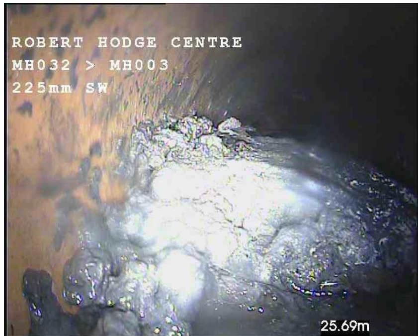
3, 25.67 m Settled deposits, coarse, 65% cross-sectional area loss
