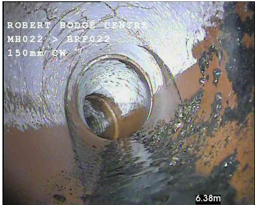
1, 6.38 m Fracture, circumferential at joint from 1 o'clock to 11 o'clock
