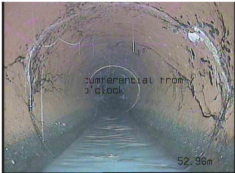
3, 00:05:30, 52.96 m Fracture, circumferential from 7 o'clock to 5 o'clock
