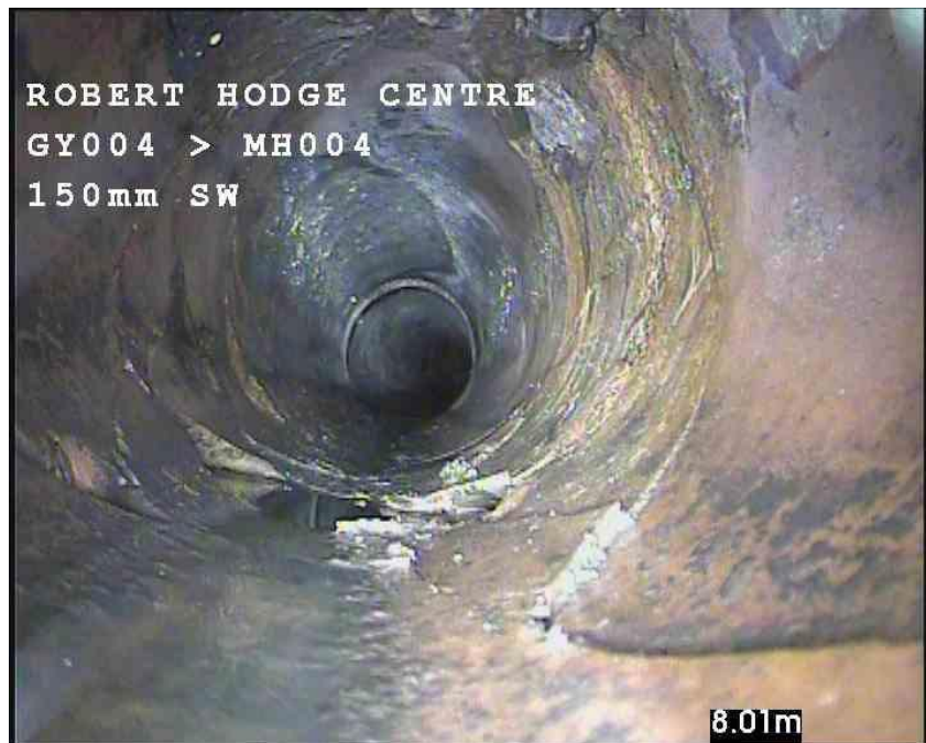
1, 8.01 m Fracture, multiple from 1 o'clock to 11 o'clock
