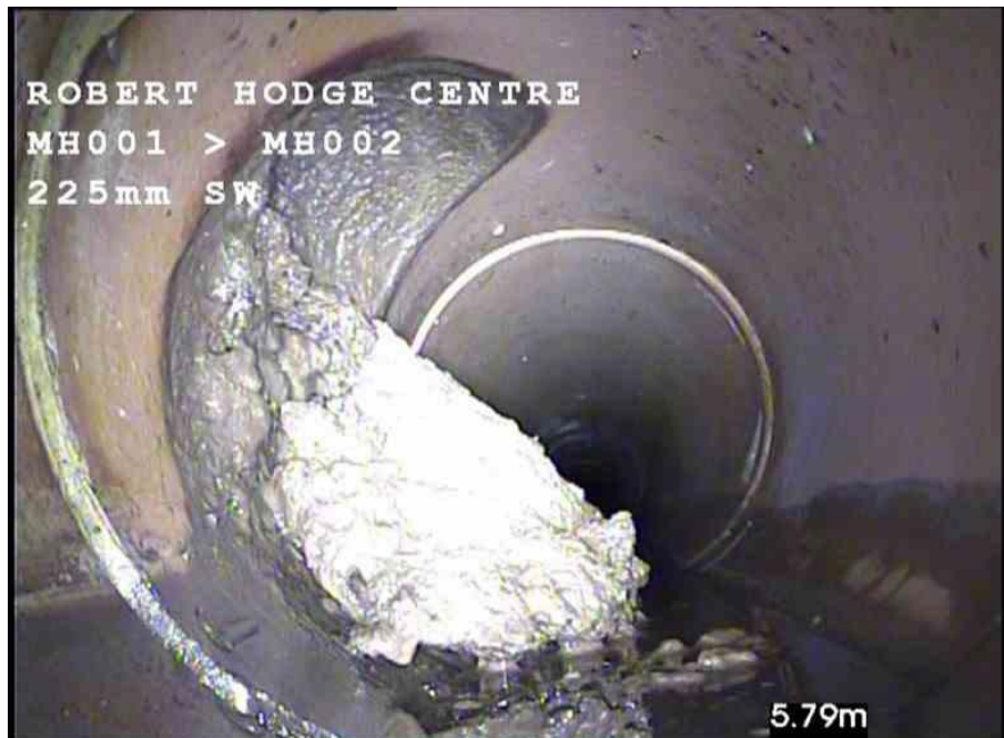
1, 5.79 m Attached deposits, encrustation from 6 o'clock to 10 o'clock, 45% cross-sectional area loss, FROM CN
