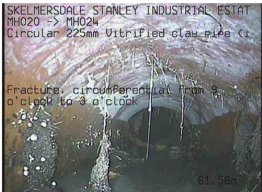
4, 00:06:30, 61.56 m Fracture, circumferential from 9 o'clock to 3 o'clock
