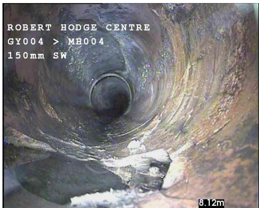
2, 8.12 m Hole in drain or sewer from 5 o'clock to 7 o'clock
