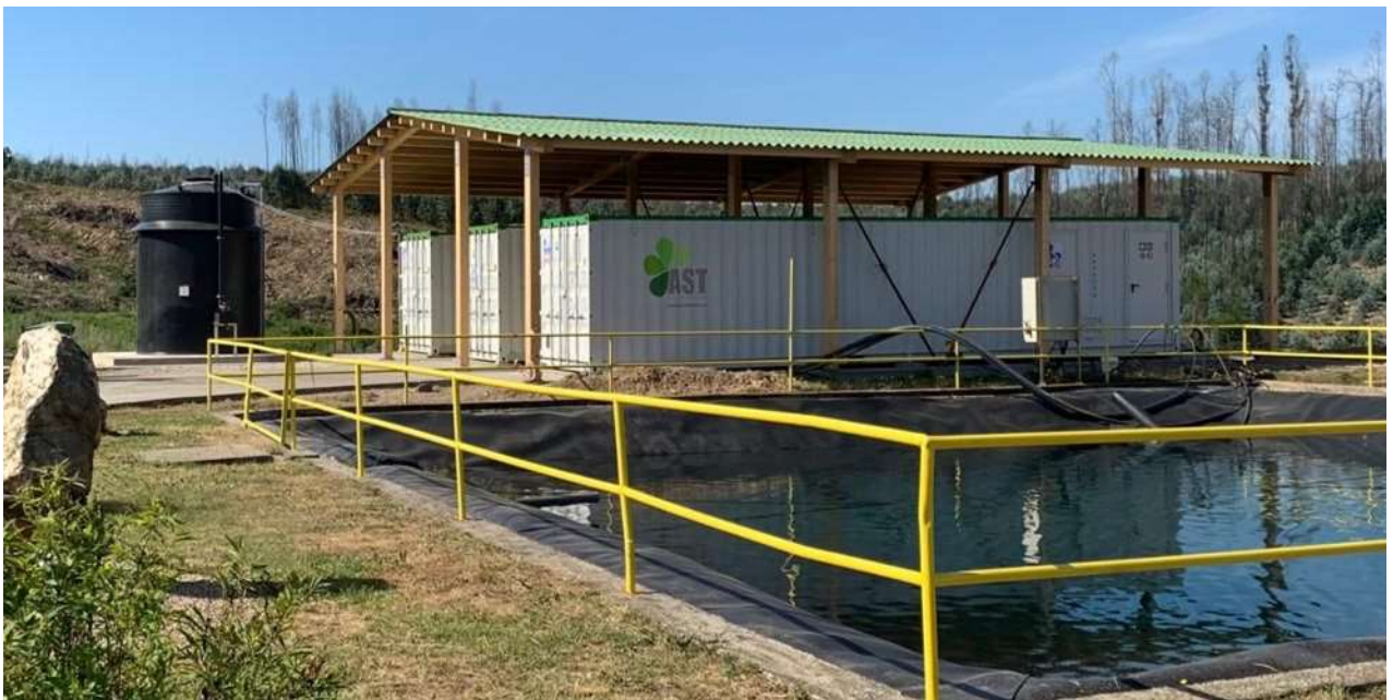
Figure 1: Reference AST - Landfill site in Tondela (Portugal) 2x200m 3 /day and 1x120 m 3 /day.
