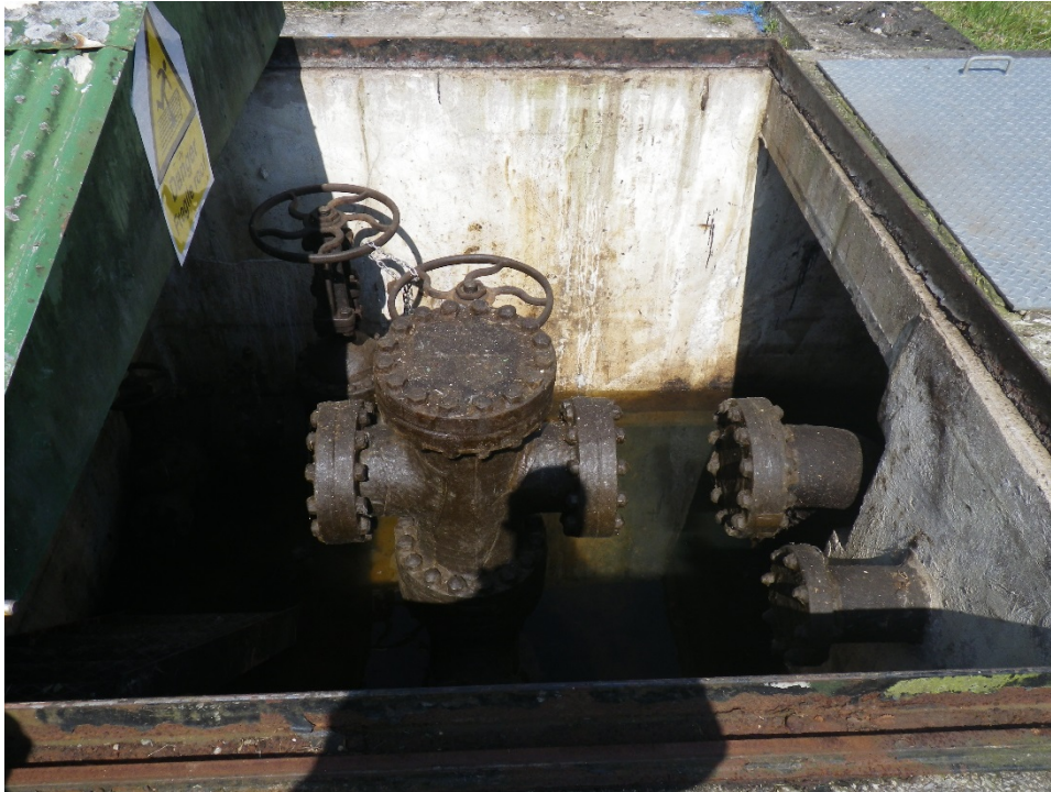
Photograph 1: Typical Well Head Chamber
