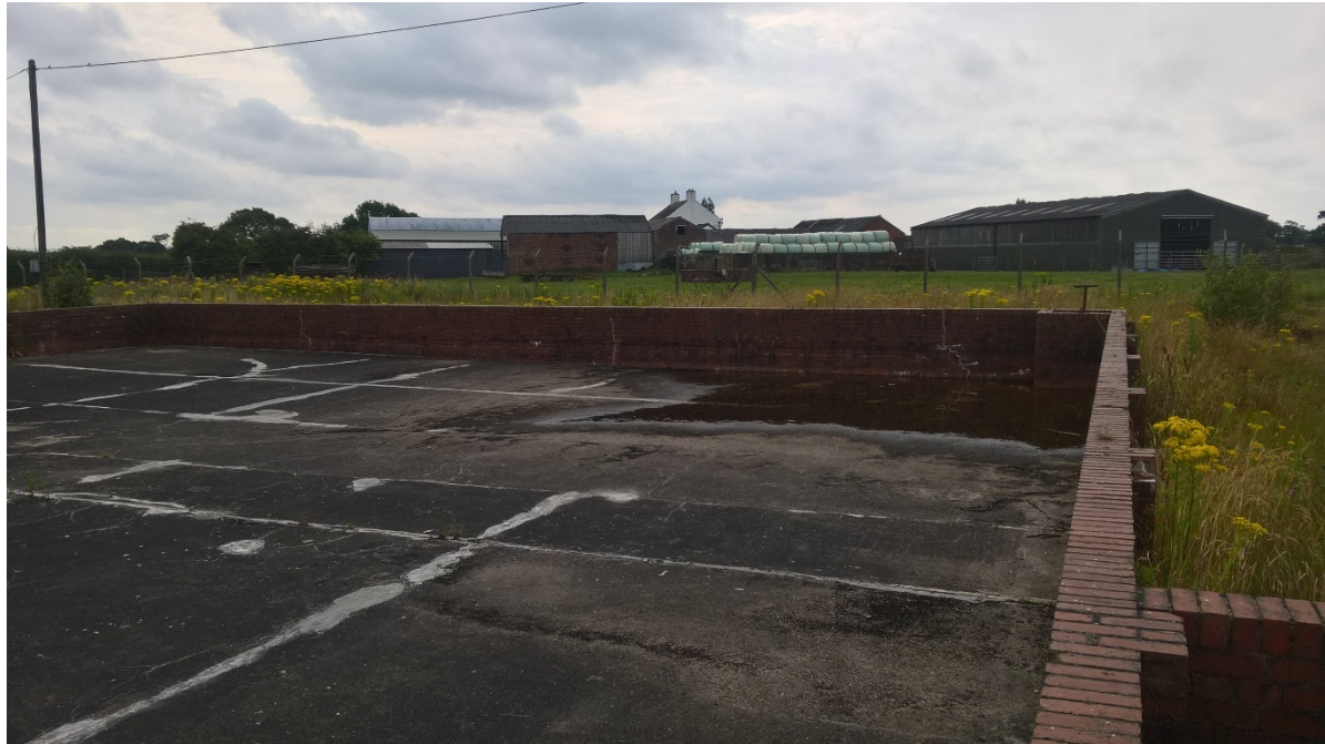
Photograph 4: Pooled surface water build-up at the point of the blocked drain in the corner of the outer bund of T171.
