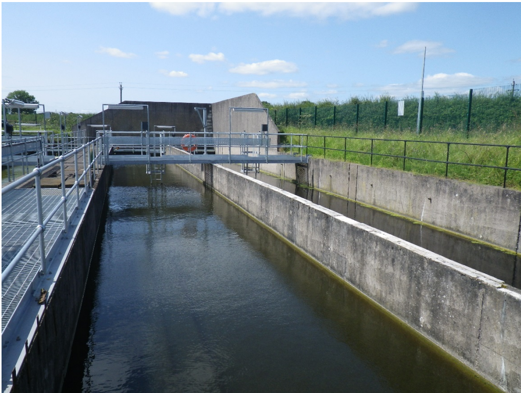
Photograph 3: Site Interceptor (showing two of four channels)
