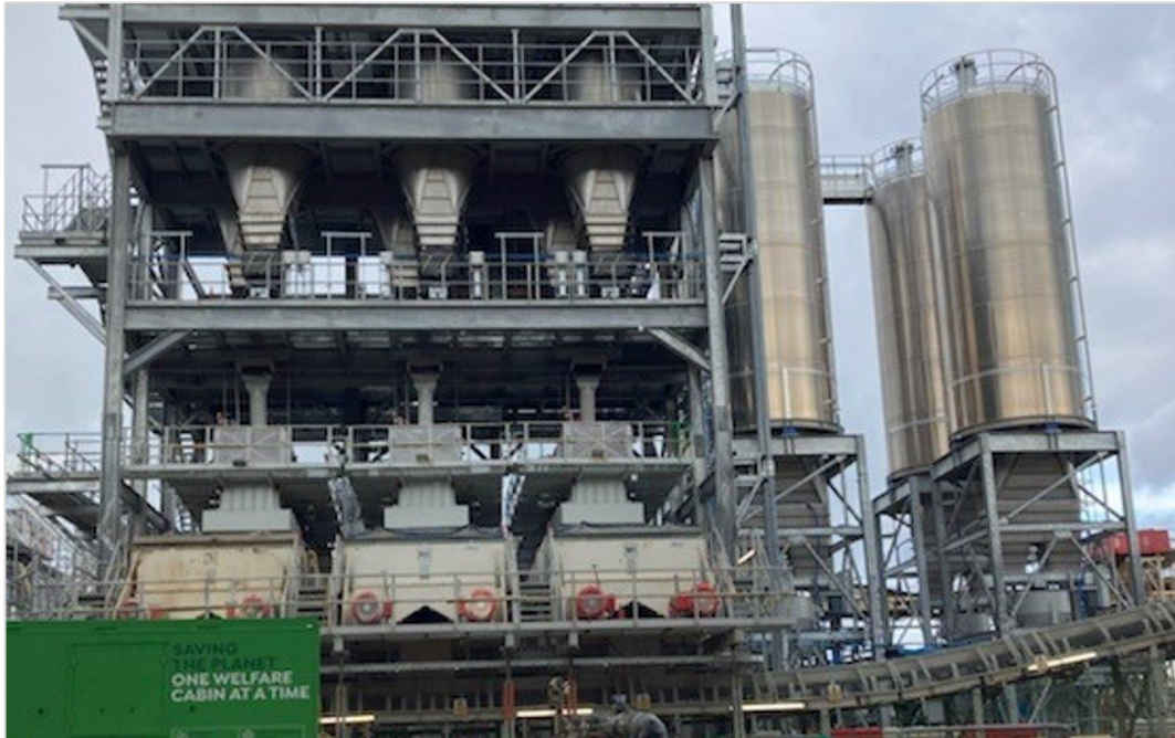
Figure 4 – Pugmills and silos
