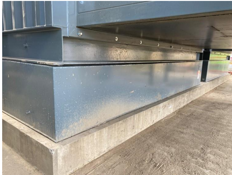
Figure 3.9 – Example bunded belly tank which sits below the generator (from EC1)
