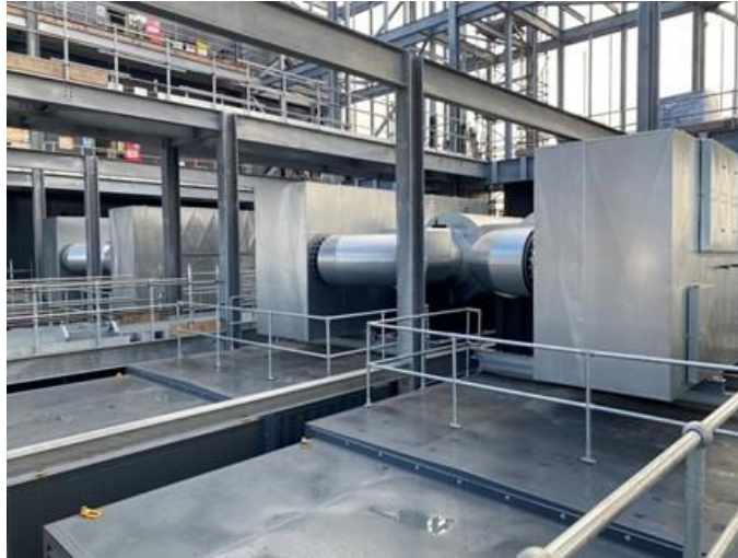
Figure 3.4 – SCR system on top of generator (Example from EC1)
