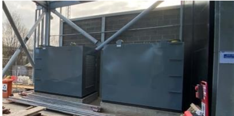
Figure 3.10 – Example of receiver tanks that feed generator belly tanks (taken from EC1)
