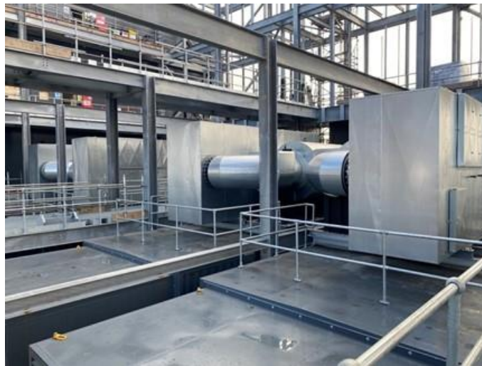
Figure 3.5– SCR system on top of generator (Example from EC1)
