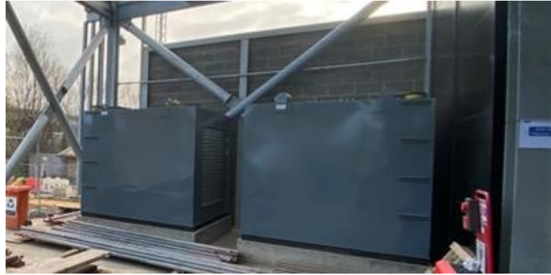
Figure 3.13 - Example of receiver tanks that feed generator belly tanks (taken from EC1)
