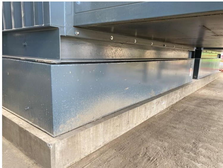
Figure 3.11 - Example bunded belly tank which sits below the generator (from EC1)
