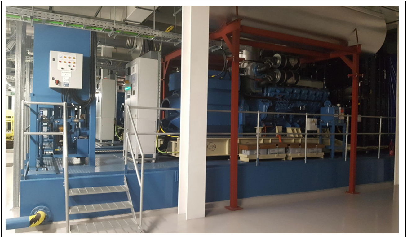
Photograph of Belly Tank set up (Generator G1/3):
