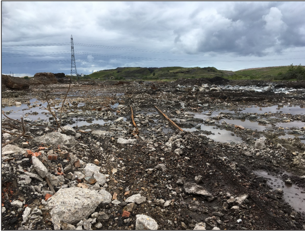
Slide 1: View looking north, taken from around the centre-southwest of the site. The photograph shows a particularly significant area of excavated material, exposing previous structures lying below the previous ground level. An old tram line, as well as large blast furnace foundations can be noted in this location.
