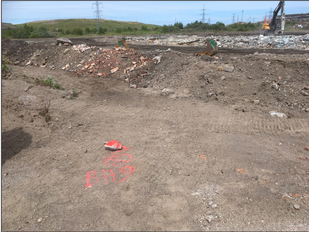
Slide 2: View looking northeast, taken from the original location of BH9. The photograph shows the demolition of large underground concrete structures in the upper right hand corner, with aforementioned areas of vegetation beyond.
