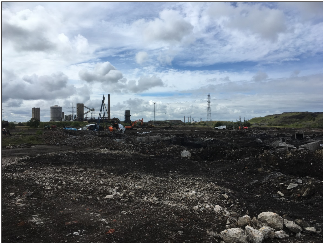
Slide 3: View looking northwest from the southeast of the site. The photograph shows a large excavation in the centre-south of the site, as well as drilling of BH12 (left of the photograph) and BH9 (right of the photograph).
