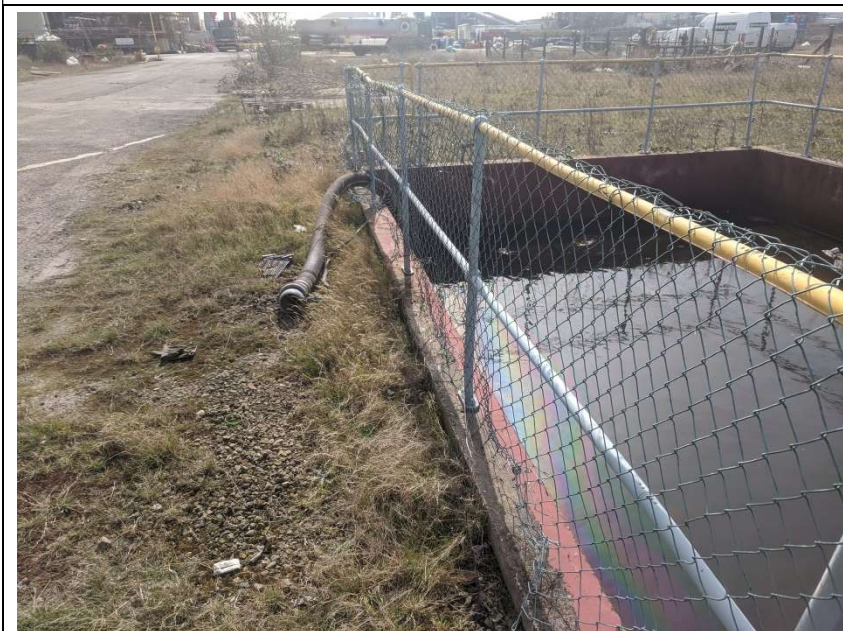
Photo 6: Pond located adjacent to the Site with vertical concrete walls and obvious surface pollution.
