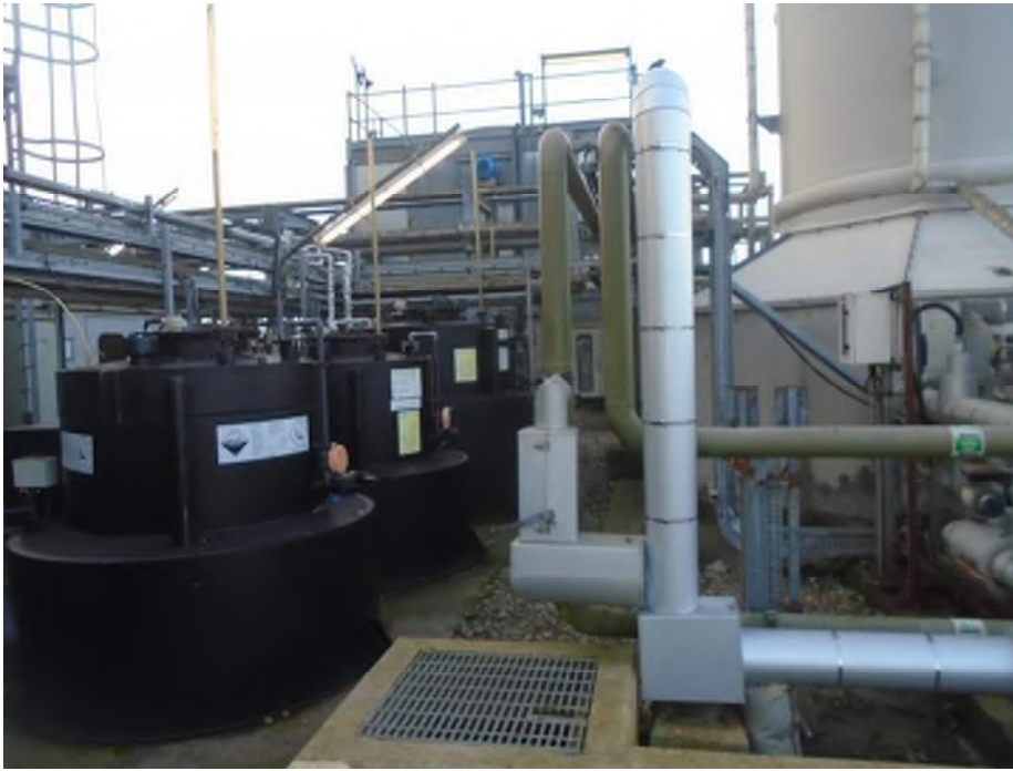
Photograph 9: Internally banded ASTs containing chemicals for water treatment (Ammonia, HCL, Drewphos, Amersite, Sulphuric Acid and Sodium Hypochlorite, 1500L to 2500L capacity).
