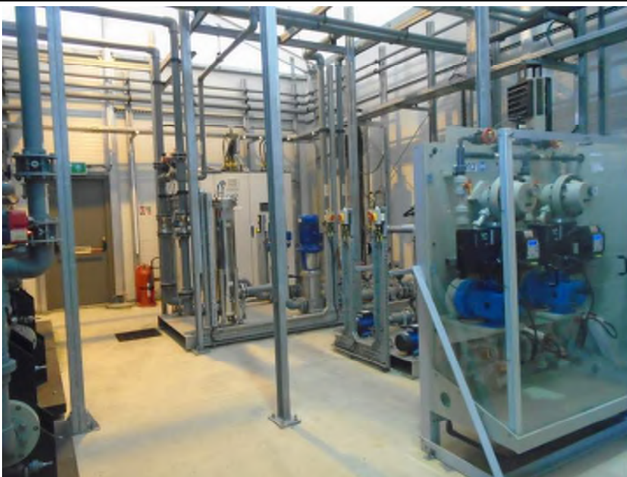
Photograph 17: General views from inside the water treatment building.
