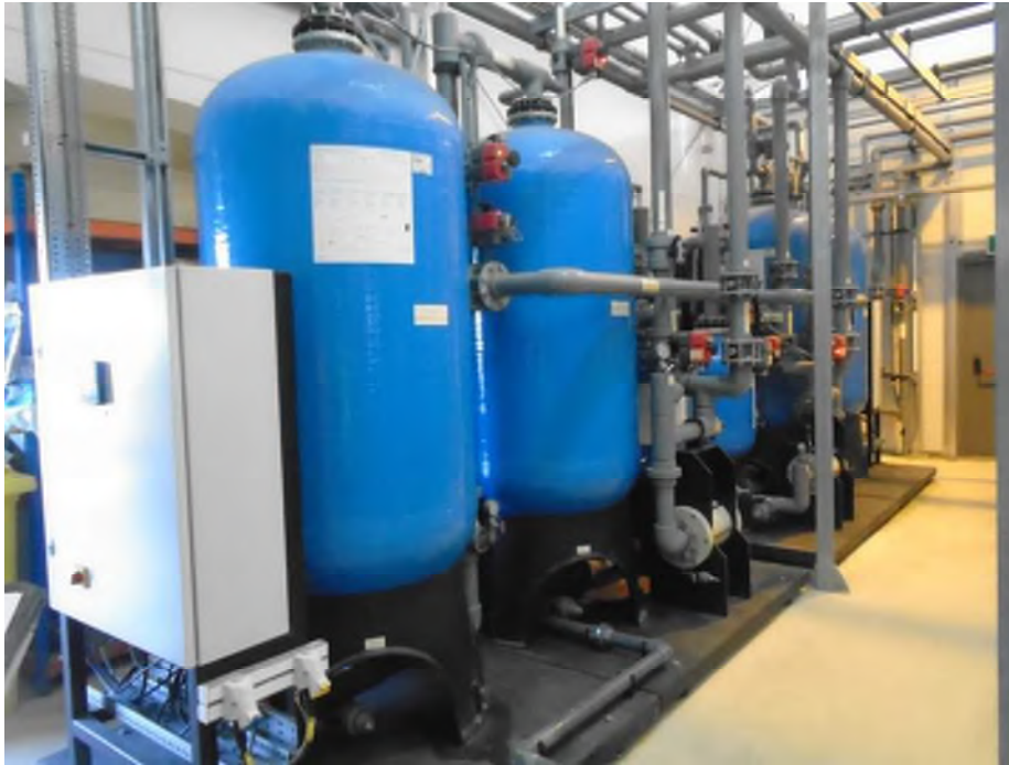
Photograph 18: General views from inside the water treatment building.
