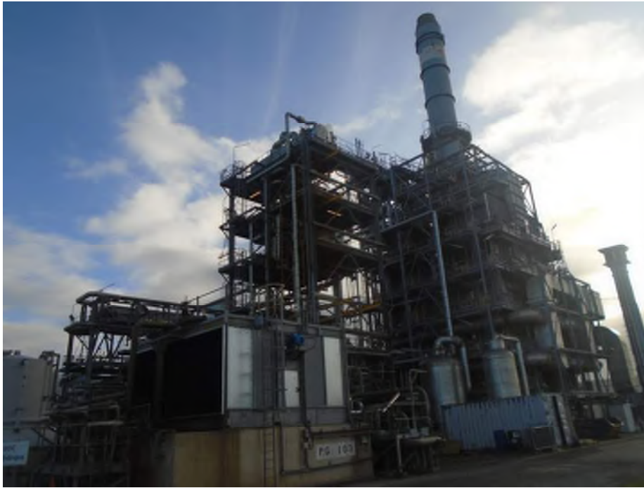
Photograph 11: General view of Site – Viewing the cooling tower (foreground) located in the northwest of the hydrogen plant.
