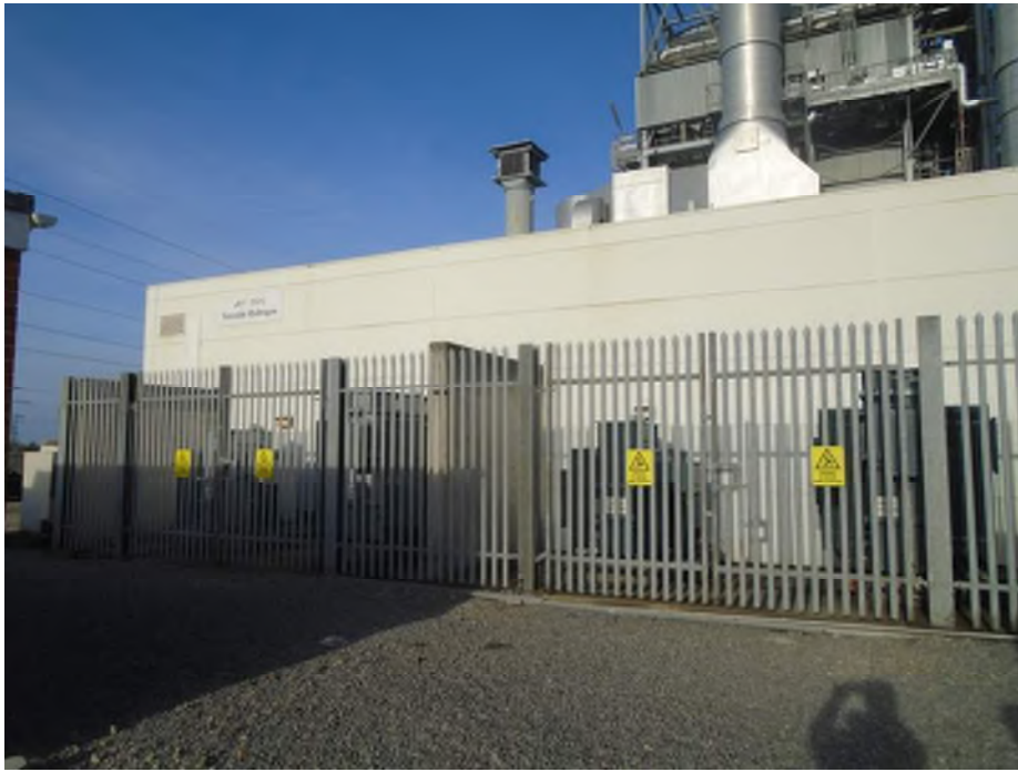
Photograph 14: Electrical transformers located immediately south of the control room, in the south of the Site.
