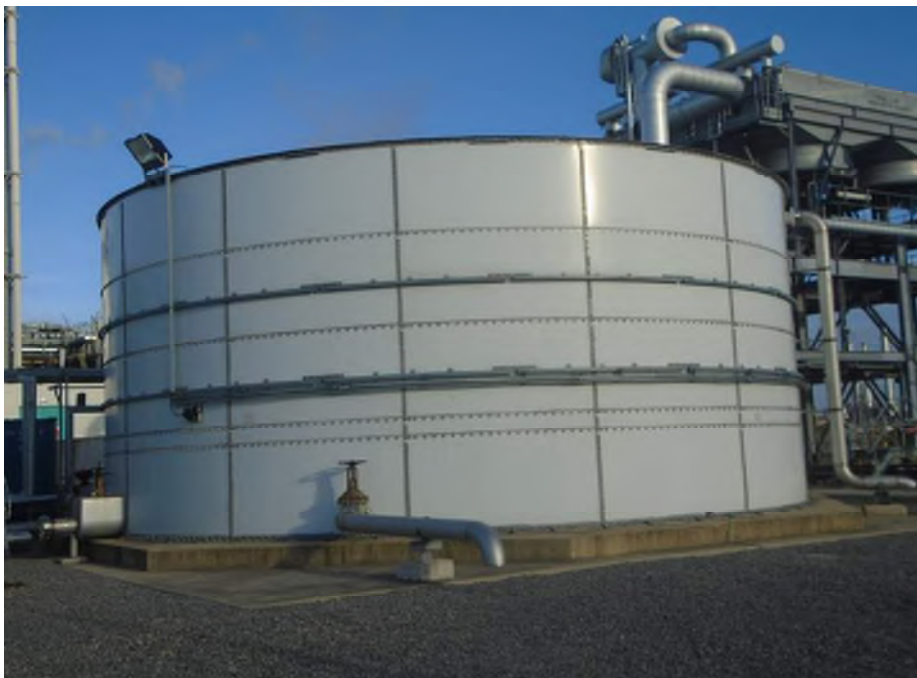
Photograph 19: 400,000L demineralised water tank.
