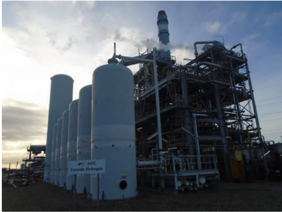
Photograph 7: General view of Site – Viewing pressure Swing Adsorption (PSA) unit in the northeast of the hydrogen plant.
