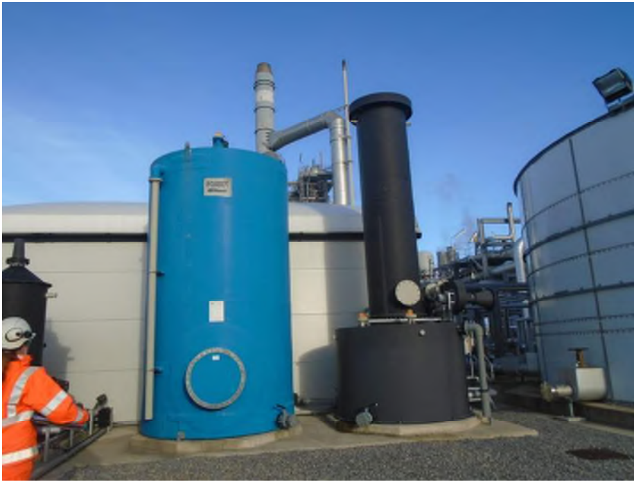
Photograph 20: 19,000L effluent tank (left of picture) and degasser tank (right of picture).
