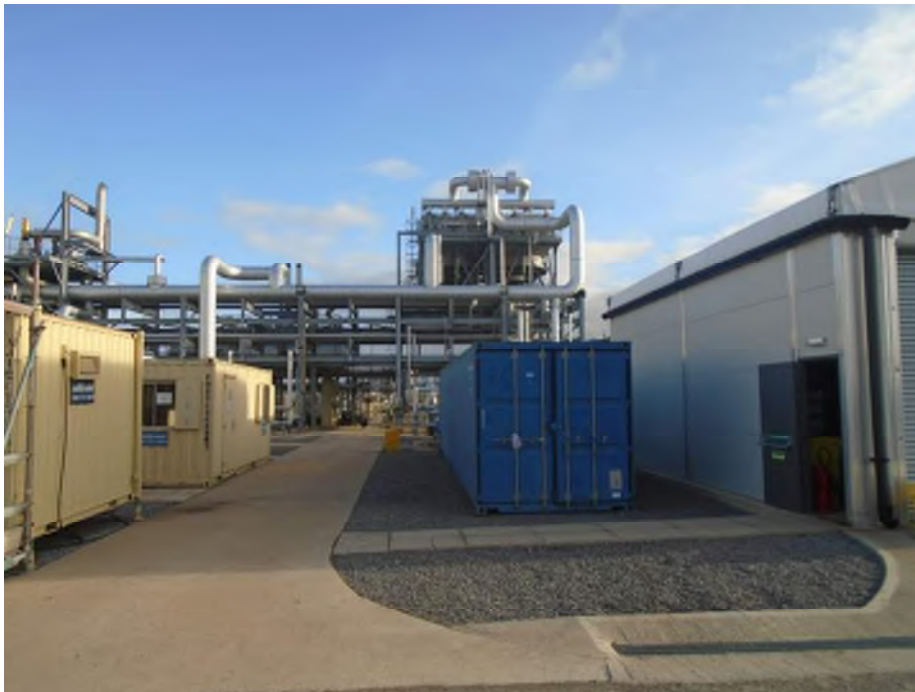
Photograph 16: Storage containers in the south of the Site (library, toilets and general storage) water treatment building to the right.
