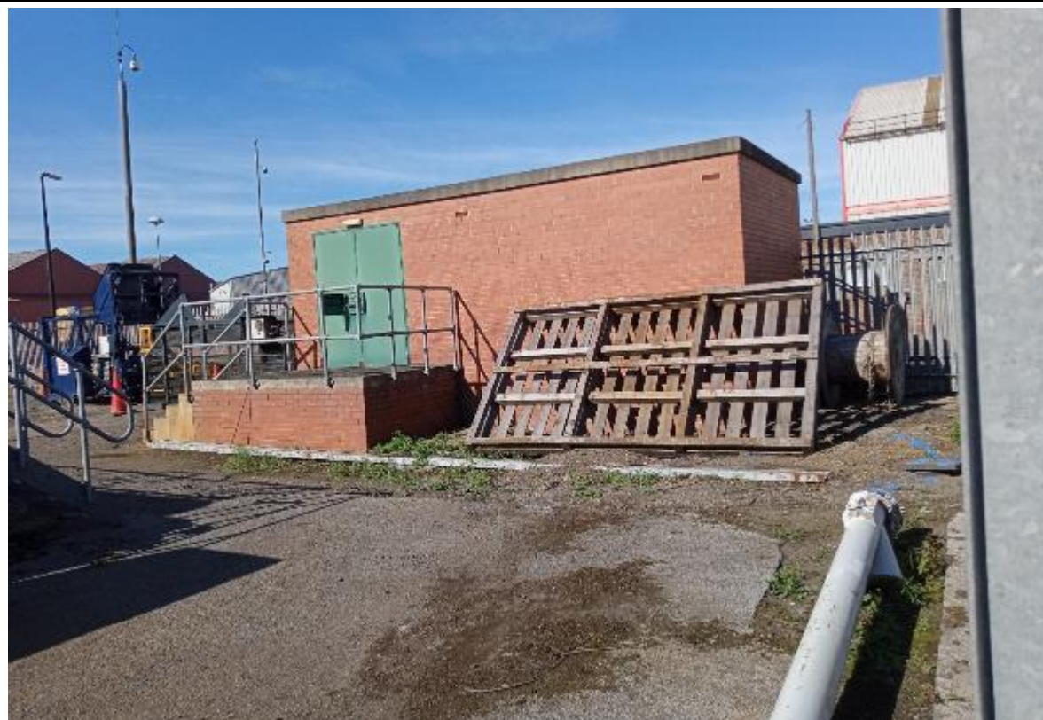
Photo looking east in the south of the site showing the smaller of the two electrical substations. Some broken concrete and sparse vegetation growth observed at surface.
