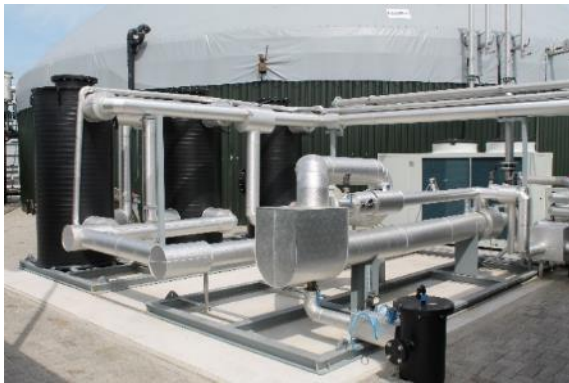
Biogas Cooling System
