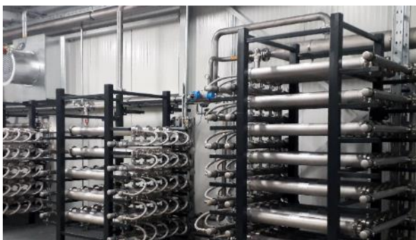
Membrane modules in a building
