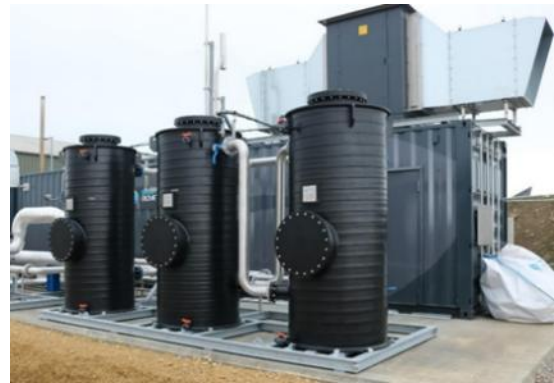
Biogas Filtration System
