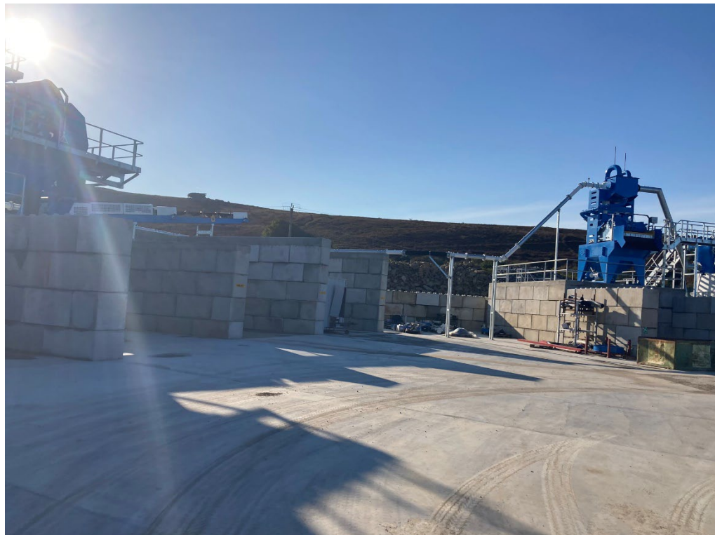
Photograph 02: View of eastern site boundary, looking in a southerly direction. New material storage bays in process of construction with soil wash plant in background. Photograph by Horizon, 11 October 2024
