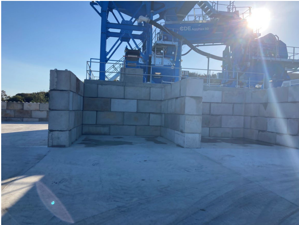
Photograph 13: View of soil wash plant in south-east corner of Site. Photograph by Horizon, 11 October 2024
