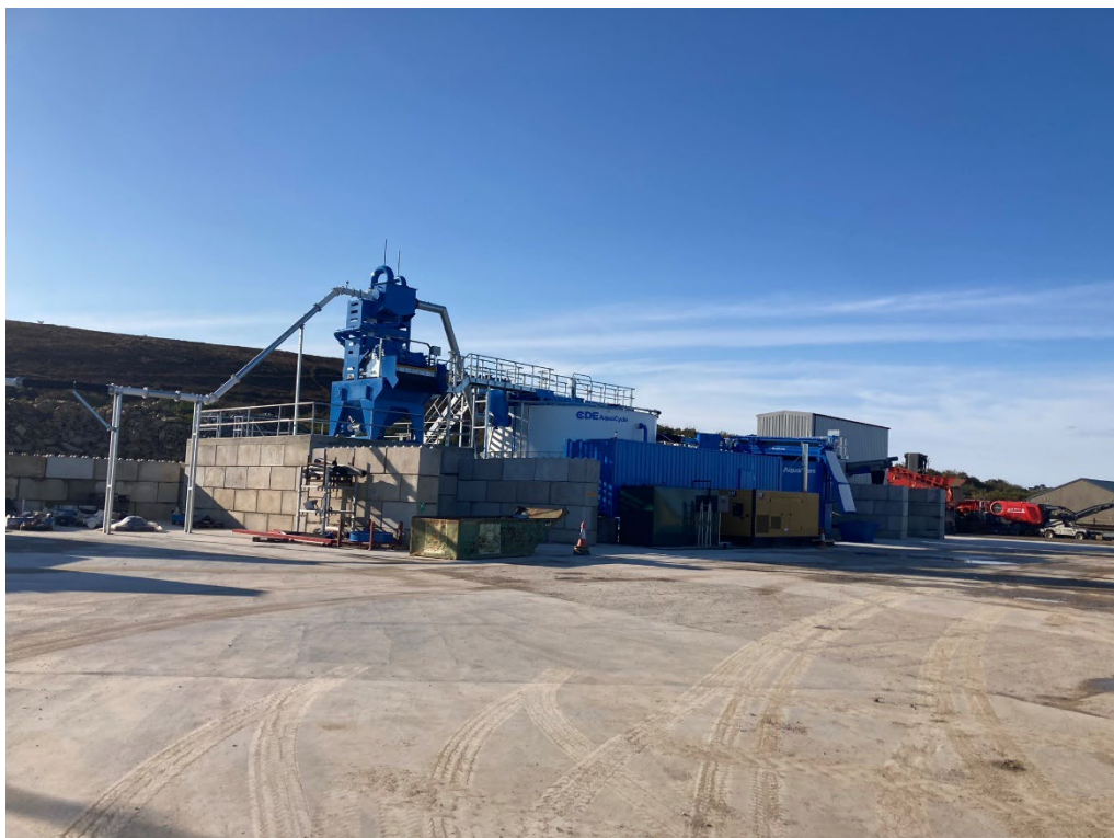
Photograph 12: View of soil wash plant along southern boundary, looking in a south-westerly direction. Photograph by Horizon, 11 October 2024
