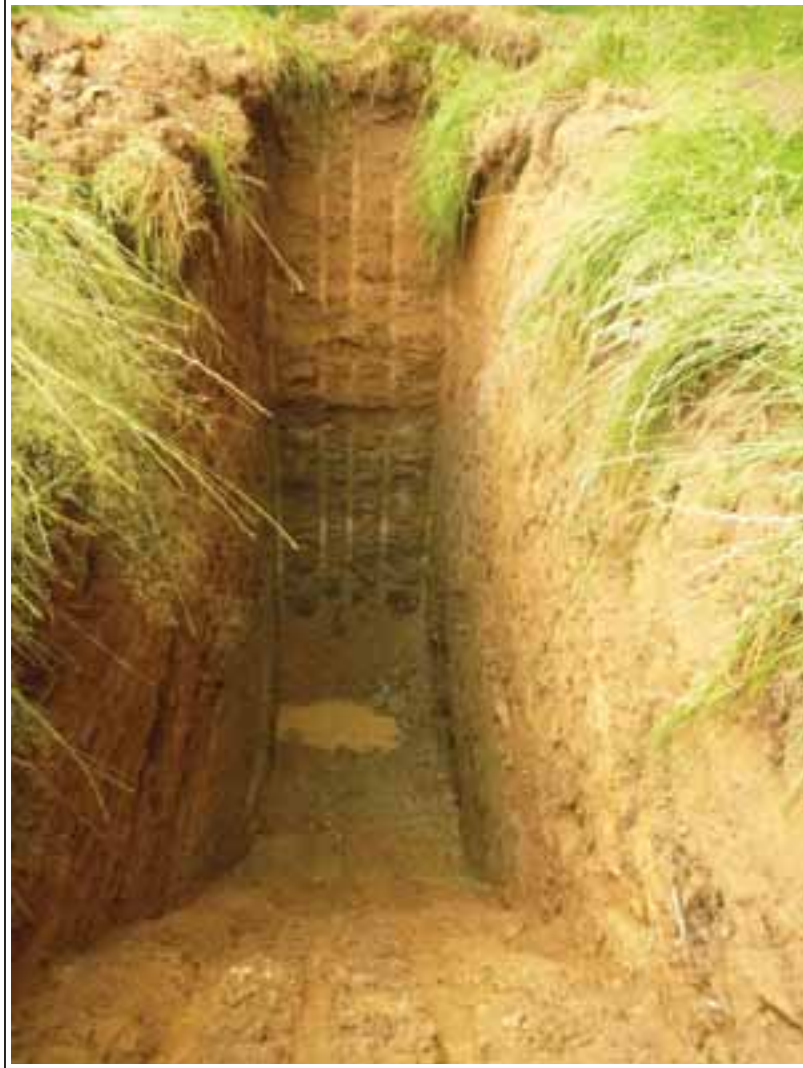
Photograph 7. Slatey gravel and groundwater seepage in Trial Pit TP10.
