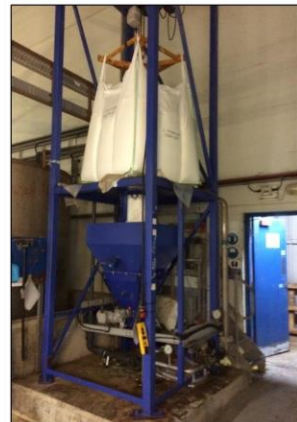
Figure 5: Polyelectrolyte hopper, dryer building
