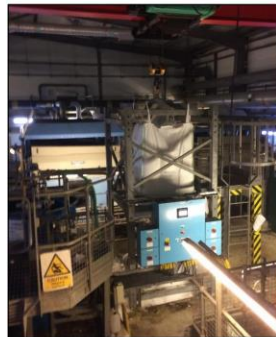
Figure 4: Polyelectrolyte hopper, inlet works building
