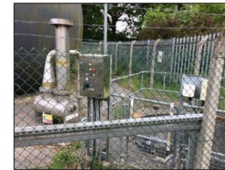
Figure 10: Gas condensate trap, gas bag area
