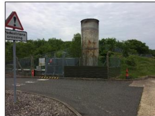
Figure 11: Flare stack compound.
