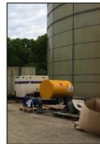
Figure 13: Portable diesel tank.
