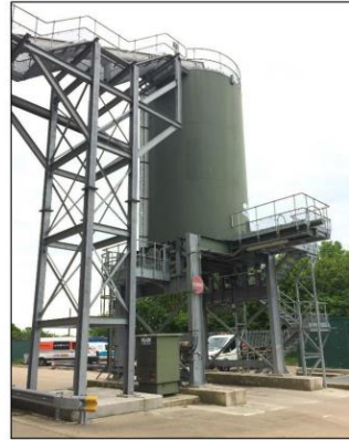
Figure 6: Post-digestion sludge cake storage silo
