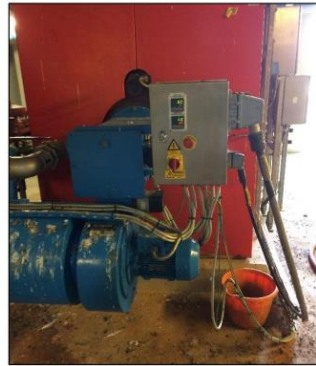
Figure 8: Water temperature controller.
