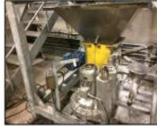
Figure 6: Polyelectrolyte hopper 1, equipment.
