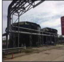
Figure 3: Post-digestion storage tanks.
