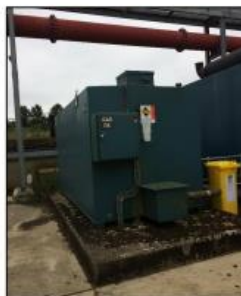
Figure 10: Diesel tank, next to tertiary treatment.
