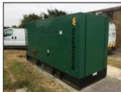
Figure 11: Diesel tank, combined with generator.
