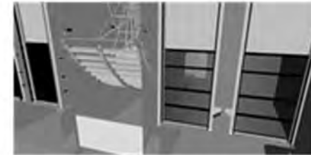
5) Detail of coarse filtration (SEF) racks leading to drum screen well
