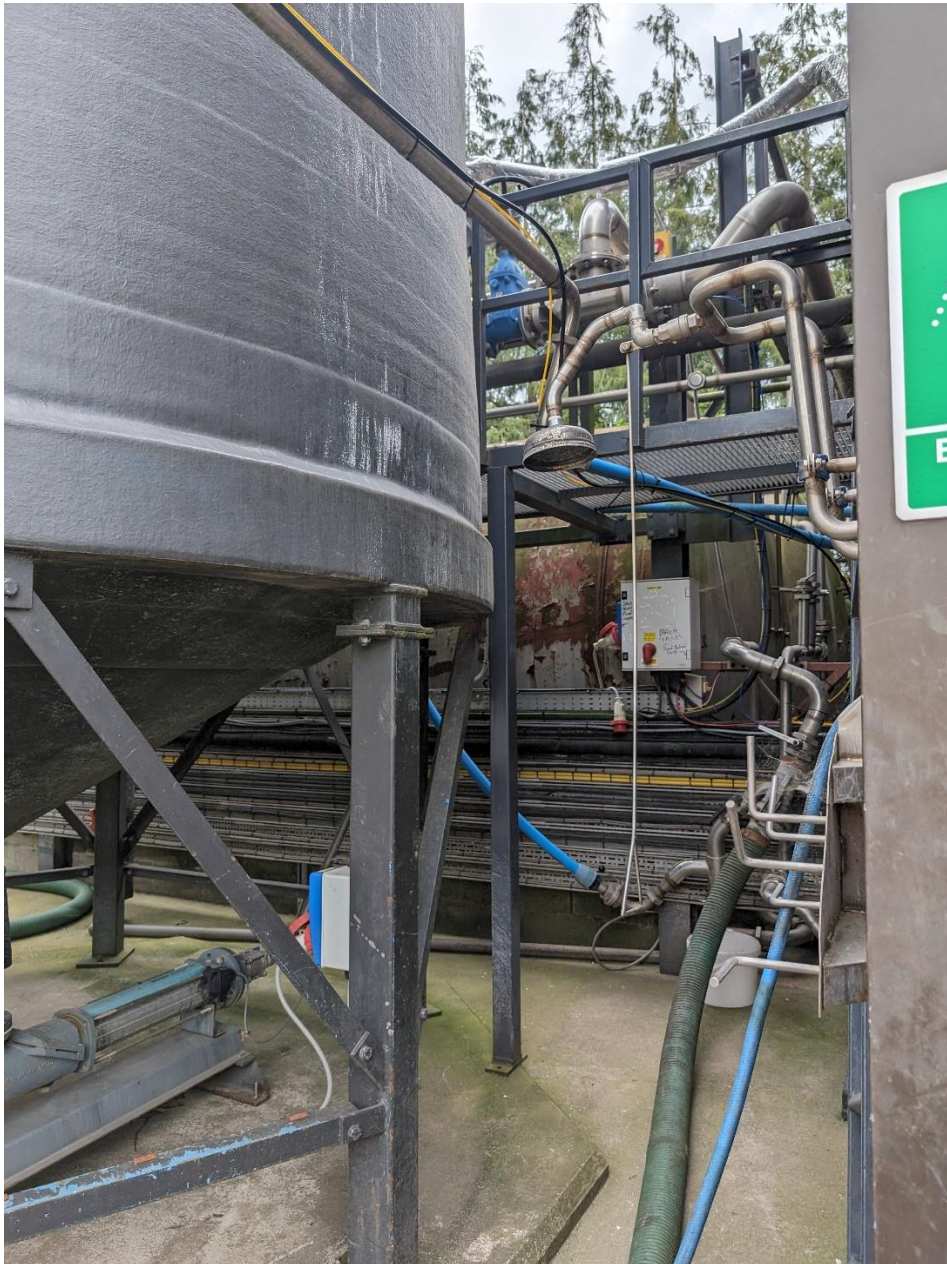
Photograph 7 –Above ground pipework Effluent Treatment Plant
