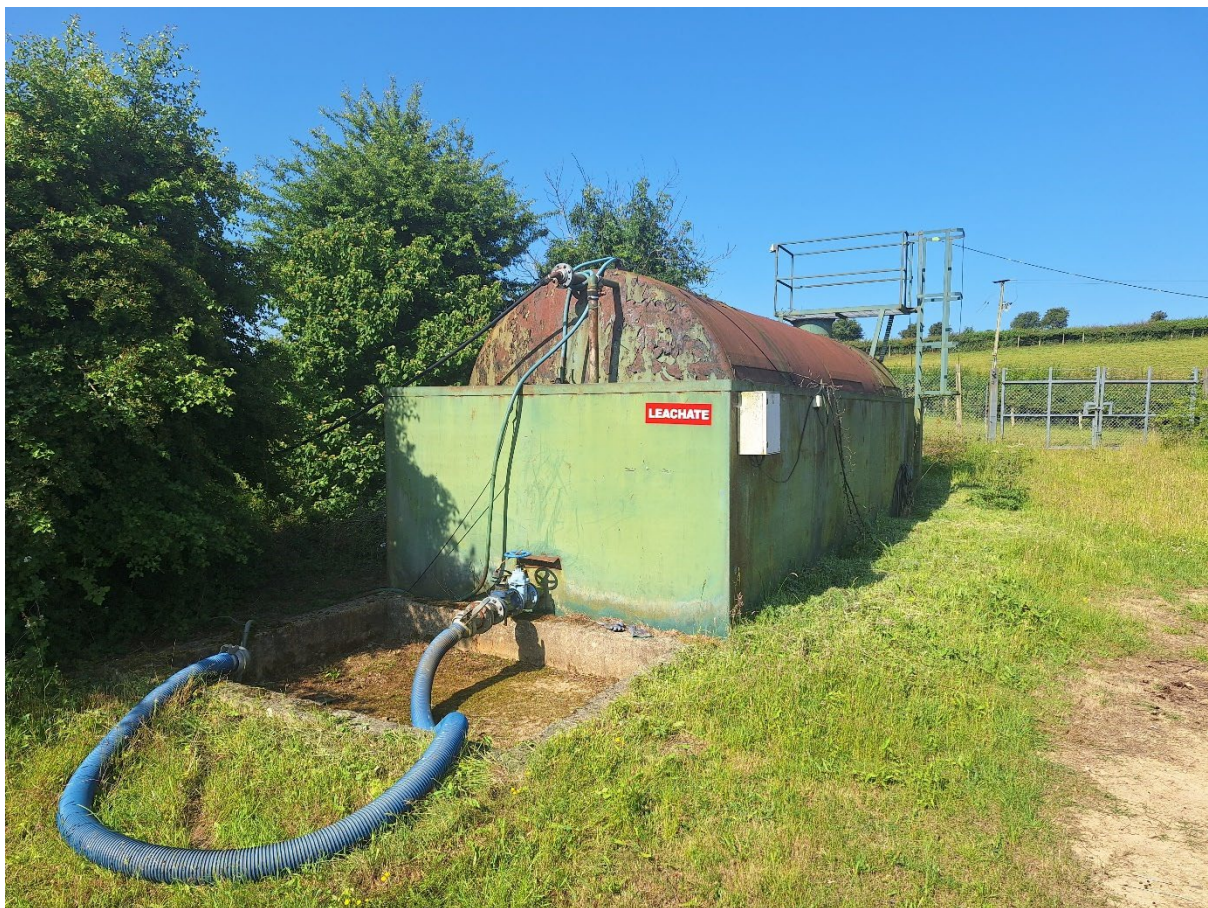
Photograph 2. Central Compound Leachate Tank (facing west)
