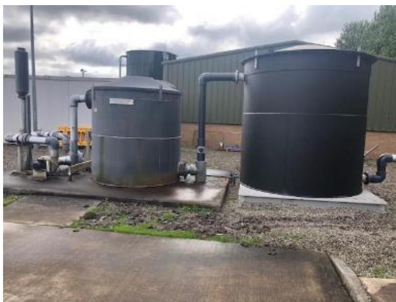
Figure 5: P6000 CIF and P3000 Peacemaker on the pre-digestion sludge blending tank
