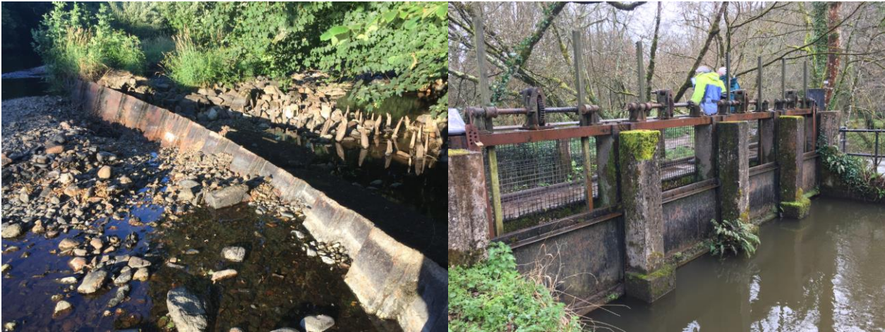
Figure 1-2 Image of the recently failed sheet piled weir (left) and large sluice gates preventing flow into the leat (right)
