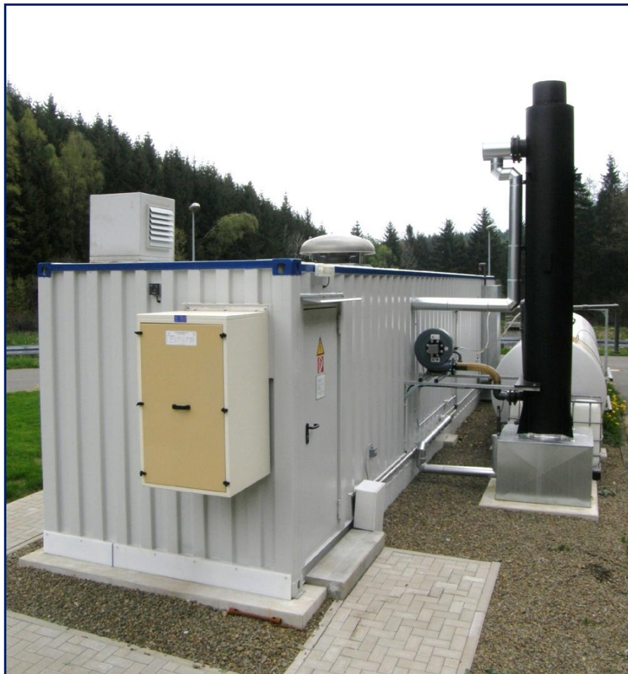
Photo: RO plant with CO 2 Stripping Tower
