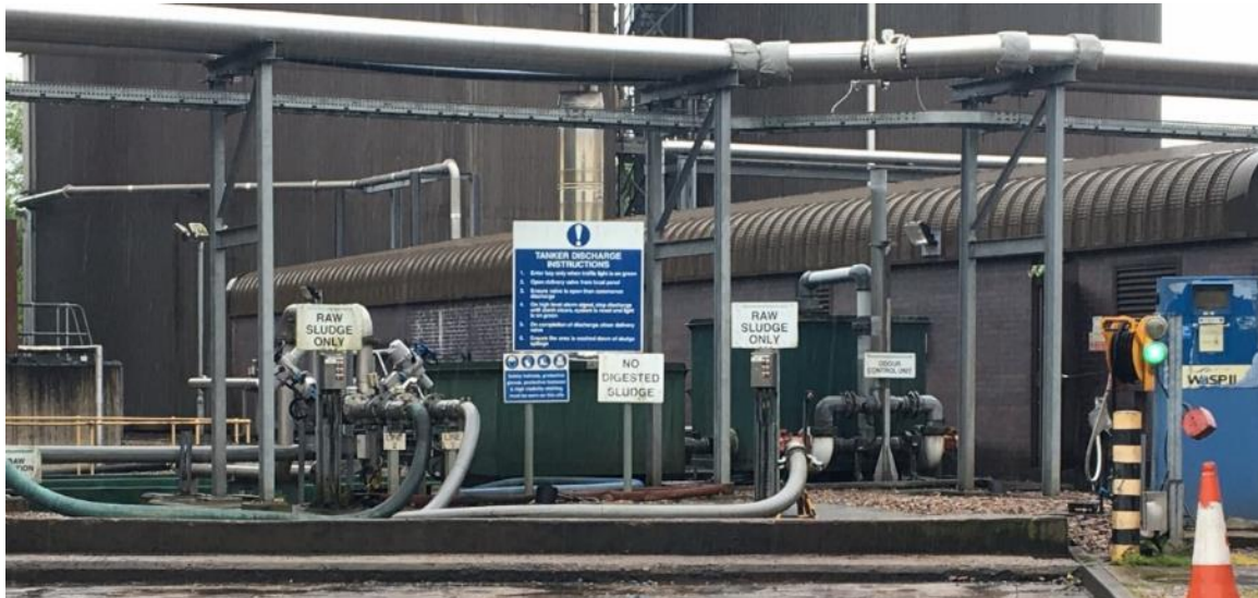
Figure 4: Raw sludge Reception tank and odour control unit
