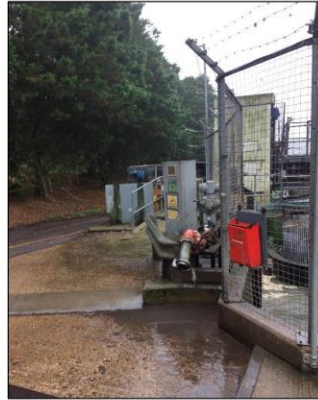
Figure 3: Cess tanker inlet.
