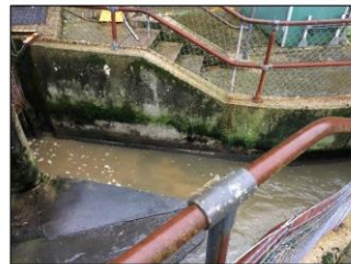
Figure 2: Inlet works, after screening.
