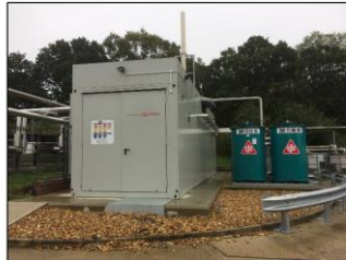
Figure 14: CHP plant, Veolia.
