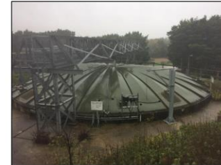
Figure 9: Post digester 2, closed.
