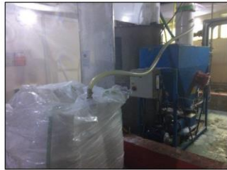
Figure 10: Polyelectrolyte dispenser 2, pump house.
