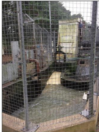
Figure 1: Inlet works, prior to screens.
