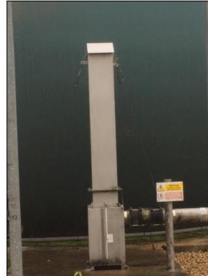
Figure 20: Gas holder compound PRV.
