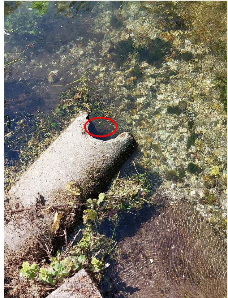
Outlet 2c: R block outlet
