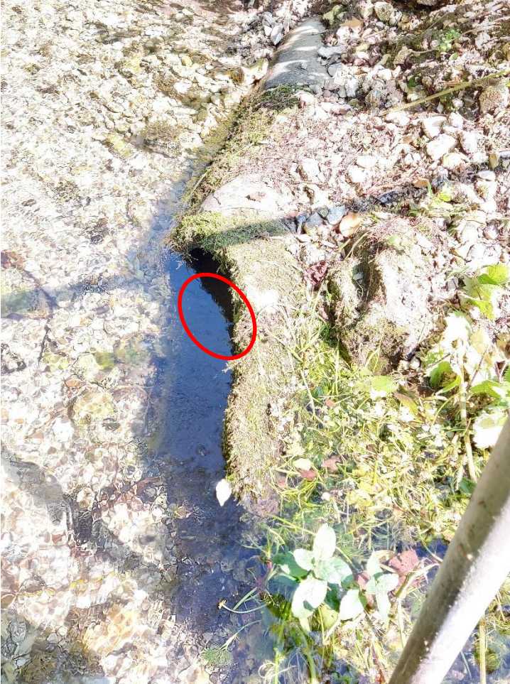
Outlet 2b: R block outlet
