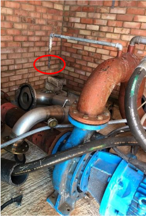
Inlet 4a: Factory BH 1
