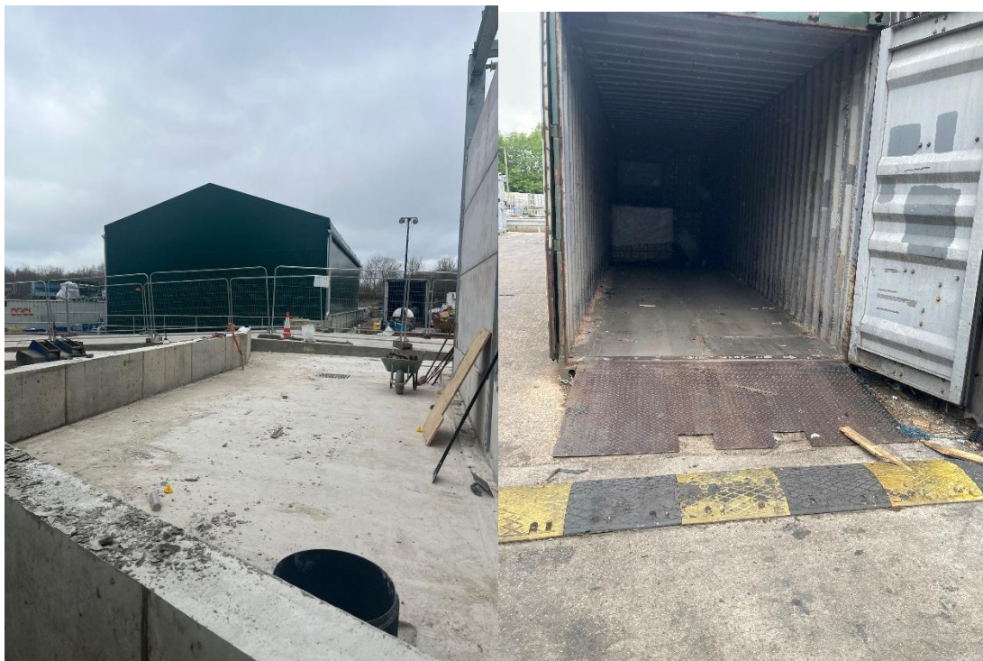
Image 20 – Tertiary containment wall and roller bund
