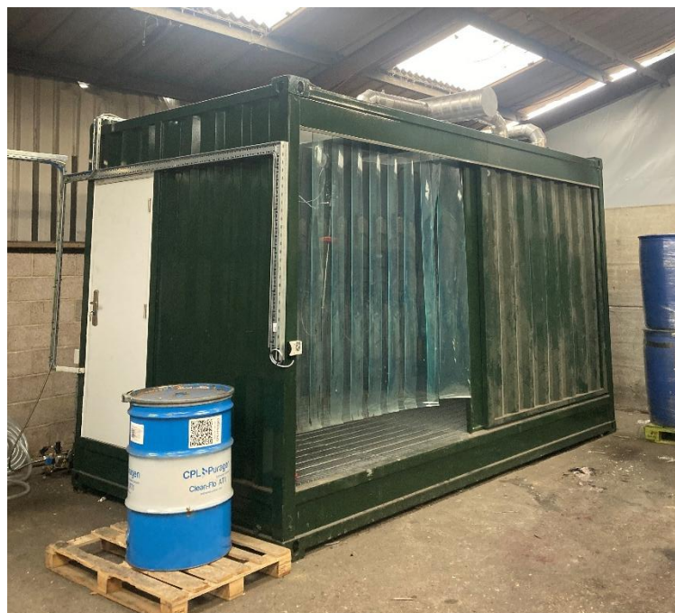
Image 17 – Bunded LEV Cabinet (A9) for Repacking & Mixing/blending & Flammable IBC decontamination
