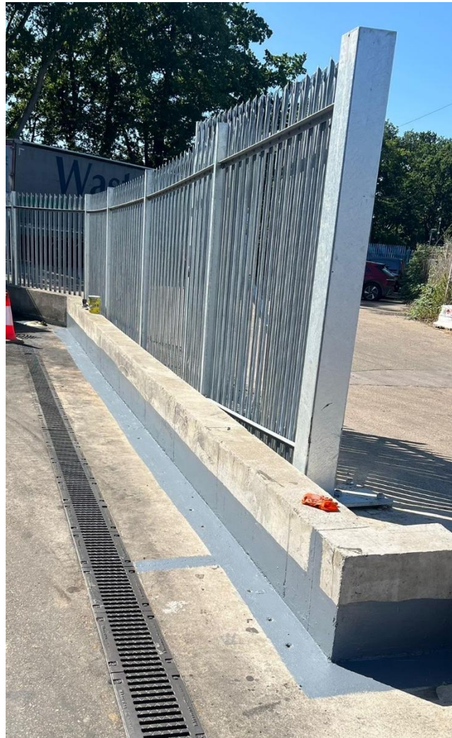
Image 11 - View from inside plastics recycling area bund towards site entrance
