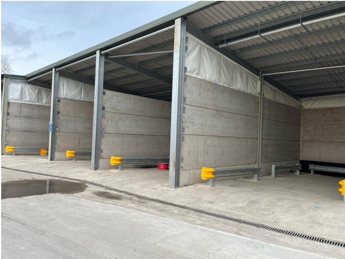
Image 16 – Views of new transfer station showing bays & Fire curtains above fire walls for combustible storage bays
