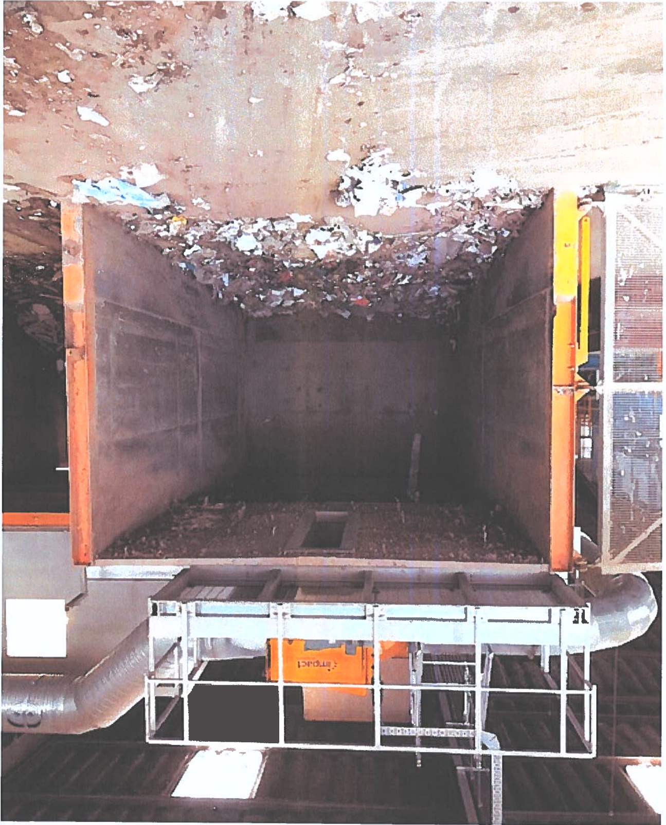
Photographic Plate(s) : 7 - Building 3, C2 Conveyor Showing blower and impact air separation
