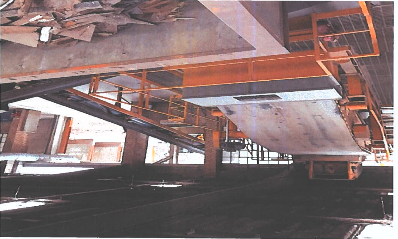
Photographic Plate(s) : 6 - Building 3, Trommel Screener Showing Production for the -6mm, destined for Area 4
