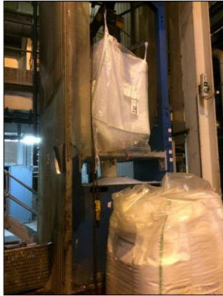
Figure 1: Polyelectrolyte hopper, dryer building.
