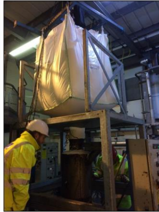
Figure 2: Polyelectrolyte hopper, next to mixing tanks.
