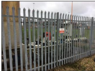
Figure 4: Flare stack compound
