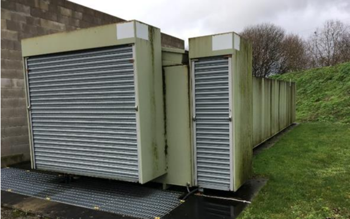
Diesel Fuel Tank
