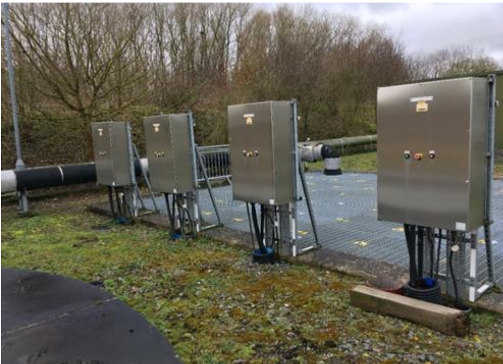
Return Pumping Station
