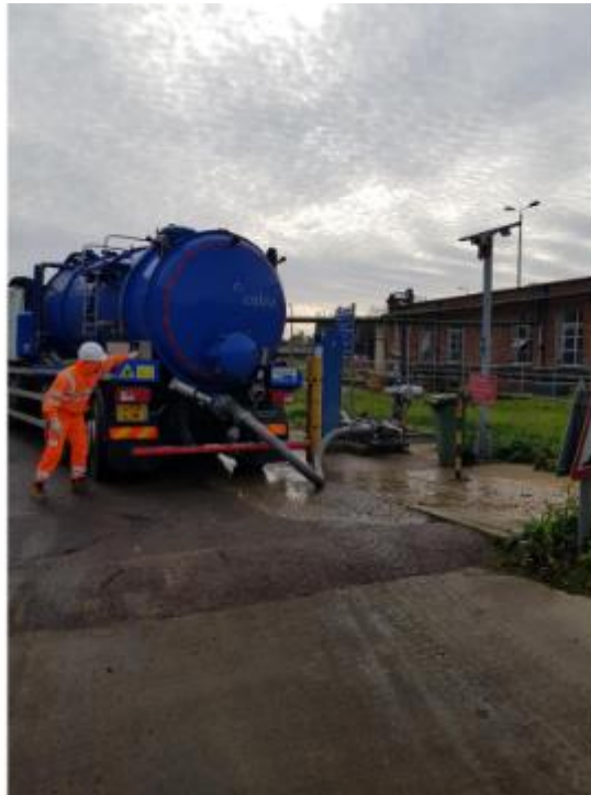
Cess/waste import area with data logger. Waste passes to the inlet for treatment.
