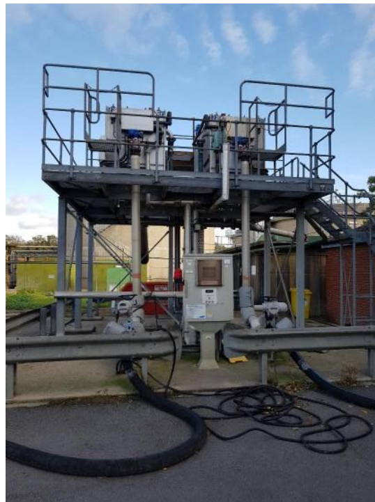
Sludge Import area and logger with two import connections. Imported sludge is first screened (at the high level) before it is discharged into the Imported Sludge Holding Tank (seen on the right).
