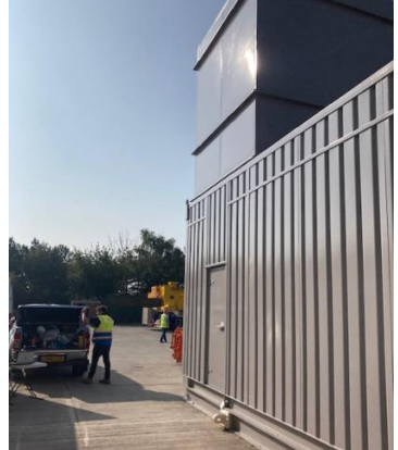
RHS of Air Outlet End
