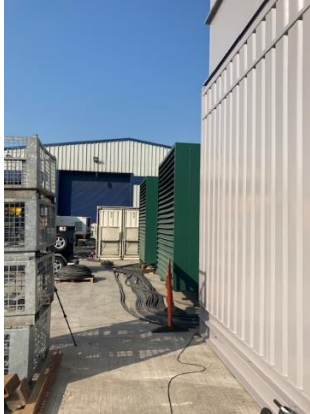
LHS of Air Outlet End
