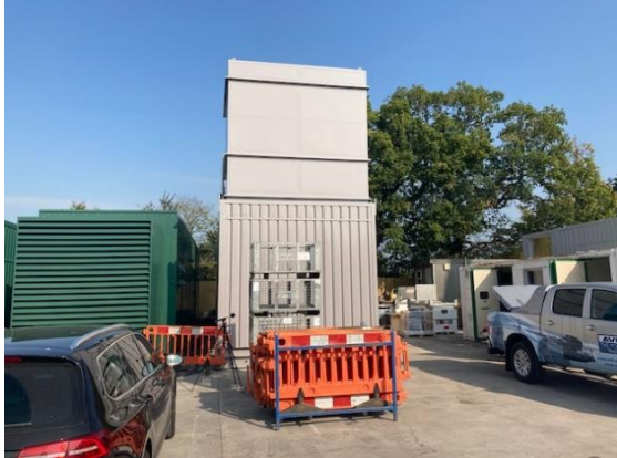
Air Outlet End
