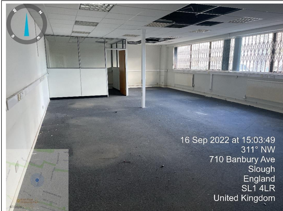
33. View of the former office area at the northern end of Bay 13
