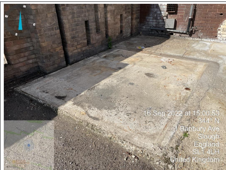
32. Evidence of a former structure (understood to be a flammable storage container) in the northwest corner of the vehicle parking area at Bay 13
