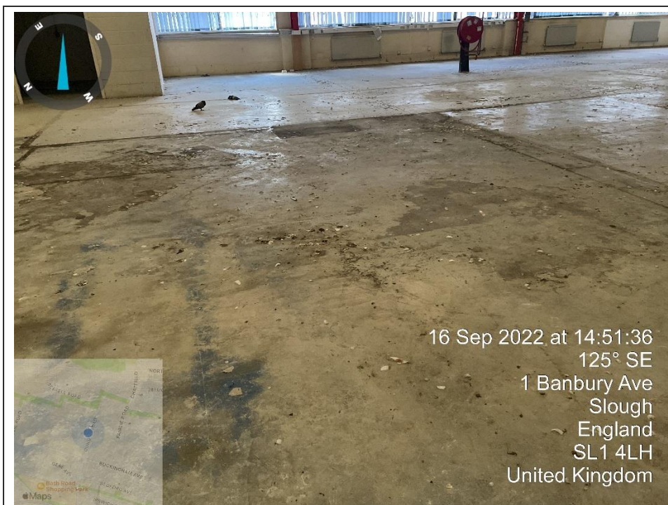
29. View of the inside of the Bay 13 warehouse showing pigeons and their droppings
