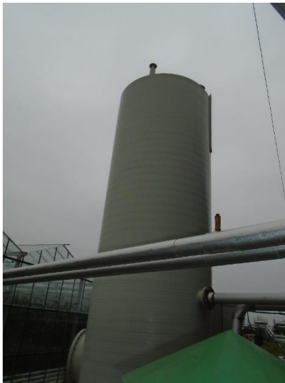
Photograph 5 – Gas Cleaning Tower
