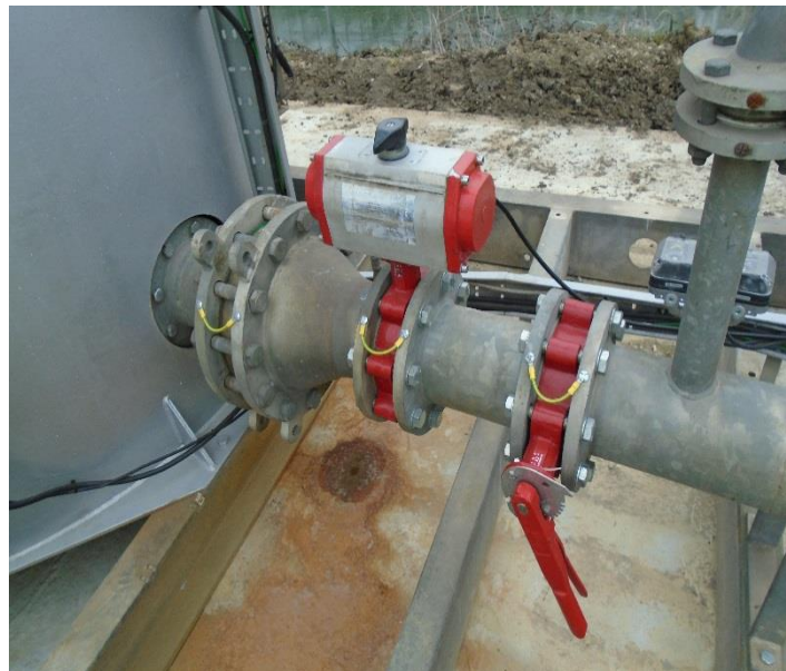
Photograph 10 – Air valve on flare stack
