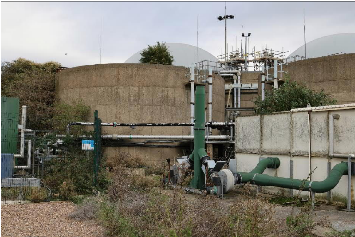
Figure 13. Digested sludge storage tanks (2 no.).
