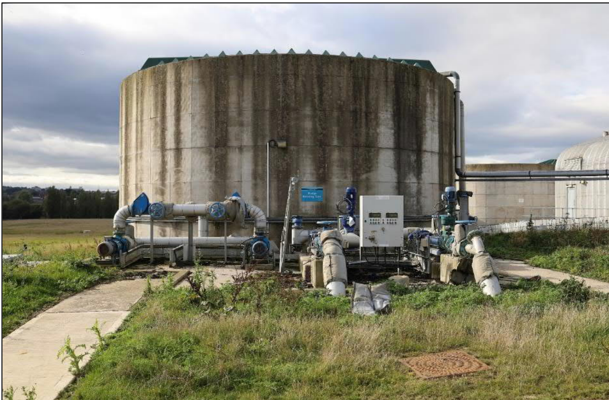
Figure 11. Digester feed tank.
