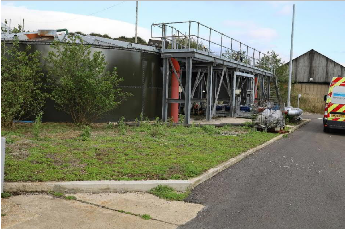
Figure 14. Liquor return balancing tanks (2 no.).
